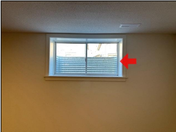
175. Difficult to operate
