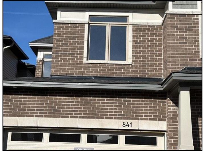
62. Debris on brick
