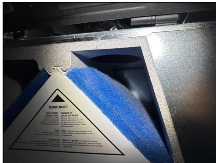
148. Dirt in cabinet
