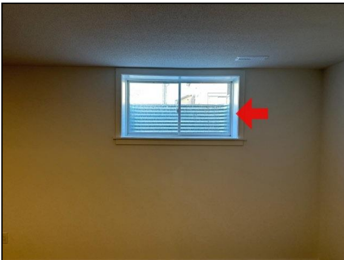
177. Difficult to operate
