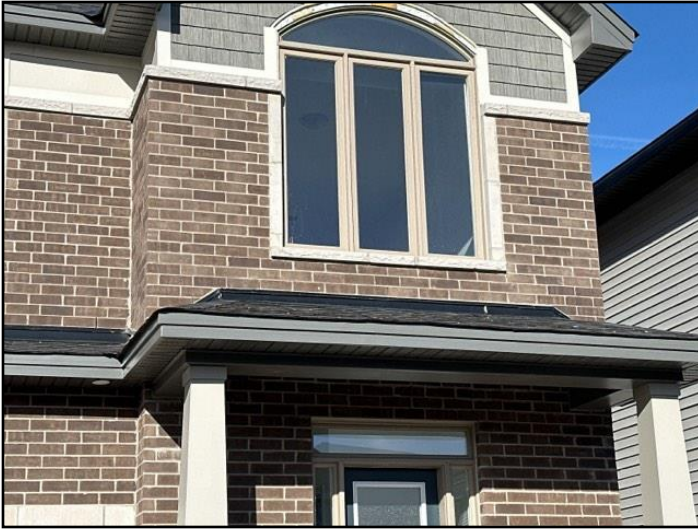
61. Debris on brick
