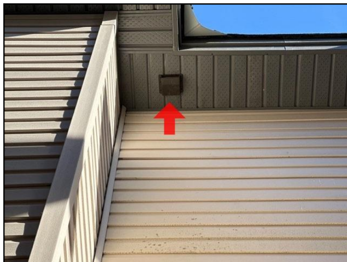
191. Clean dryer vent
