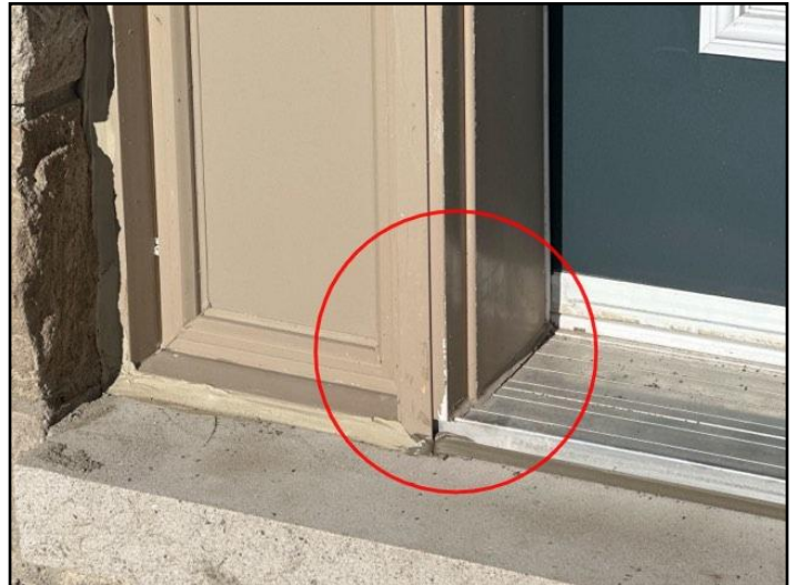
91. Damaged, cracked or loose
