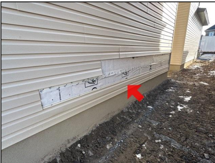
26. Loose or missing pieces
