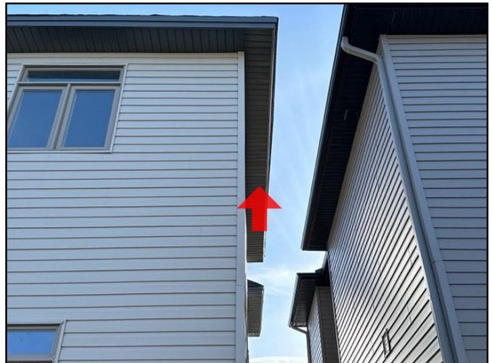
189. Does not discharge to exterior
