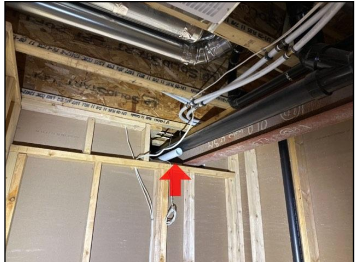
135. Not well secured
