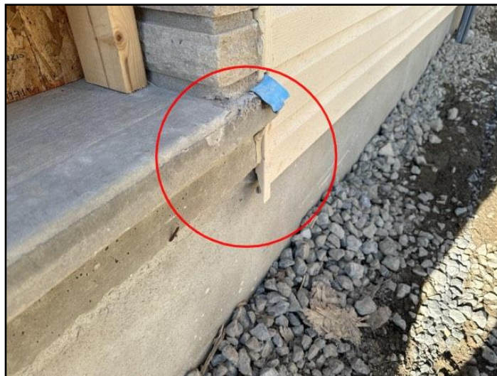
23. Caulking missing or ineffective
