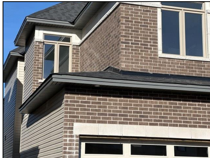
63. Debris on brick
