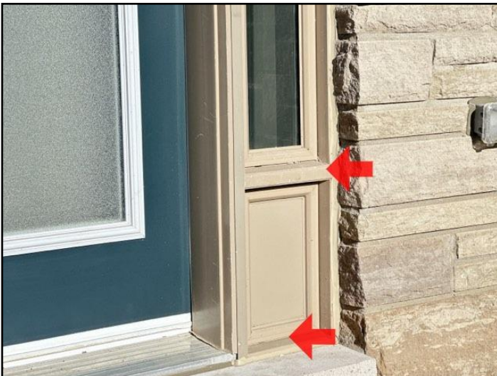
94. Damaged, cracked or loose
