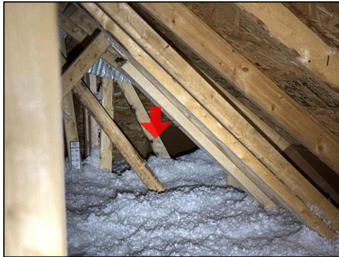
150. Gaps or voids
