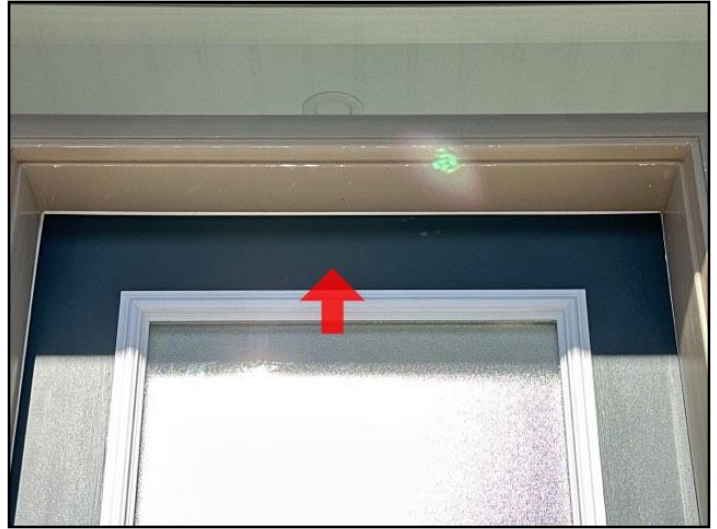
93. Damaged, cracked or loose
