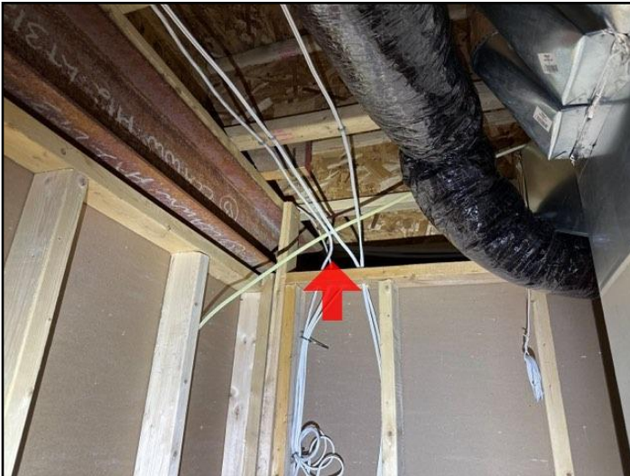
134. Not well secured
