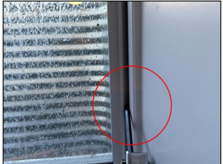
176. Difficult to operate
