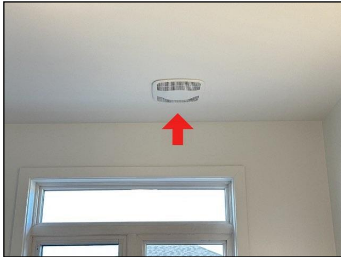
190. Does not discharge to exterior
