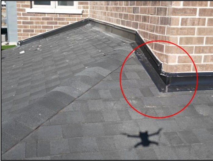
10. Damage, loose, open seams, patched
