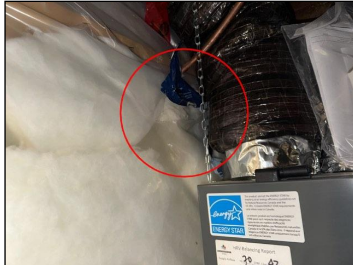
152. Loose, sagging or voids
