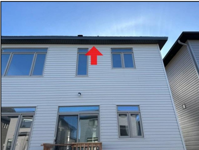
188. Does not discharge to exterior
