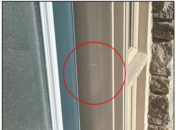
95. Damaged, cracked or loose
