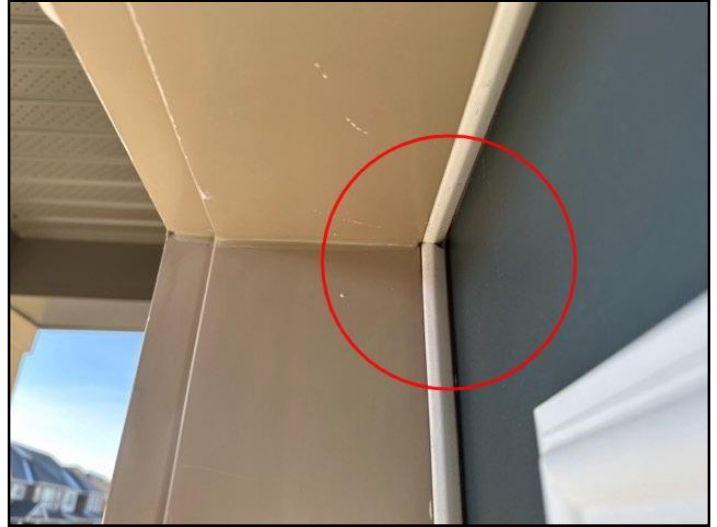
187. Weatherstripping missing or ineffective
