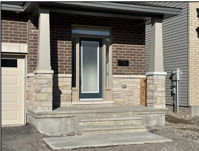
59. Debris on brick
