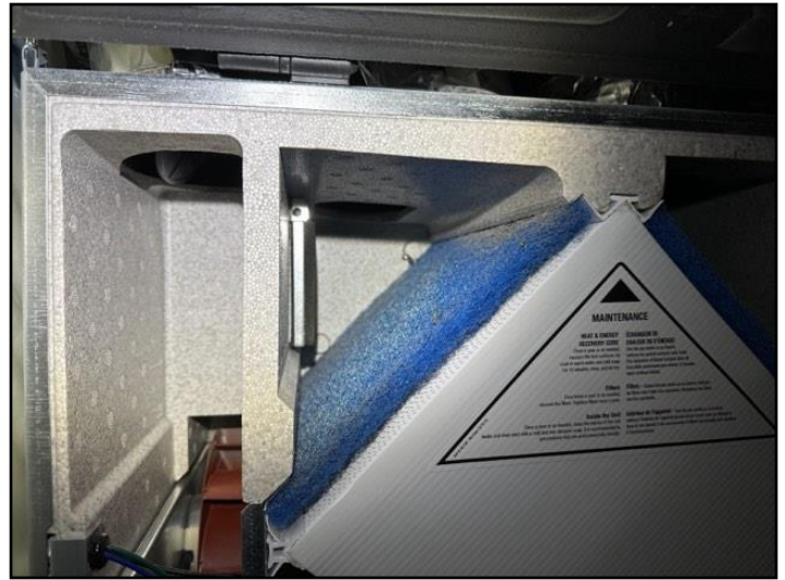
147. Dirt in cabinet
