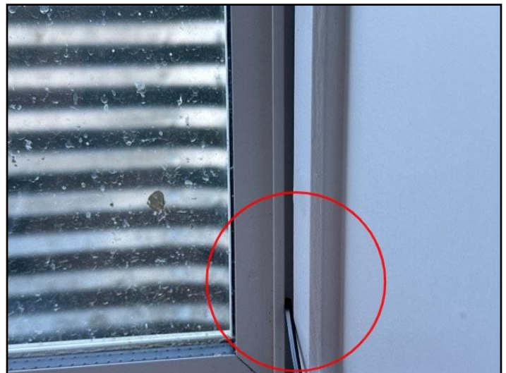
178. Difficult to operate
