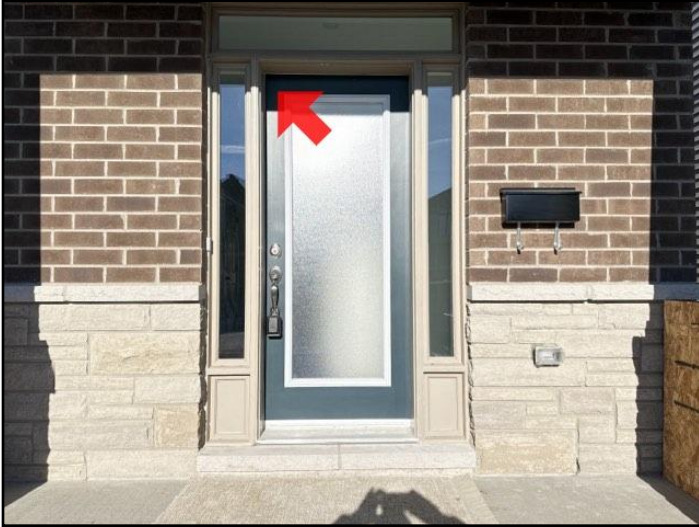
186. Weatherstripping missing or ineffective
