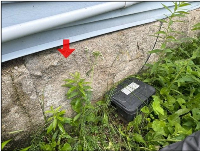
107. Spalling, crumbling or broken material
