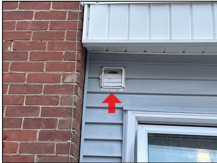
212. Clean dryer vent
