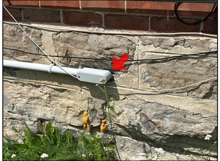
21. Caulking missing or ineffective
