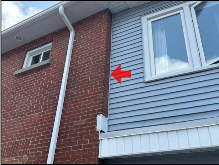
32. Caulking missing or ineffective
