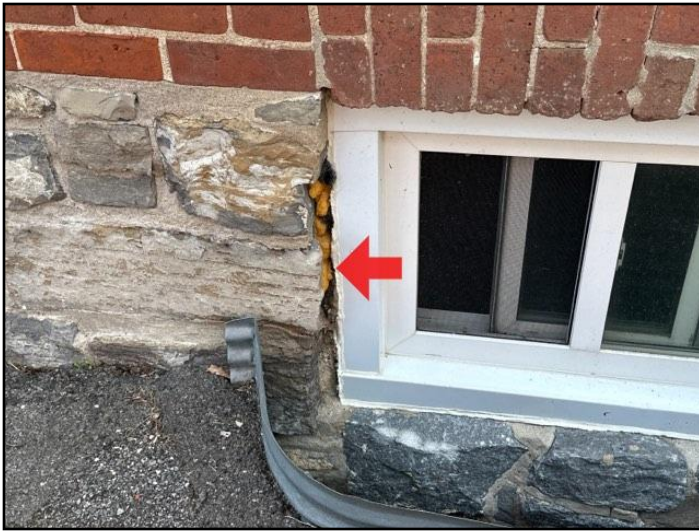
28. Caulking missing or ineffective
