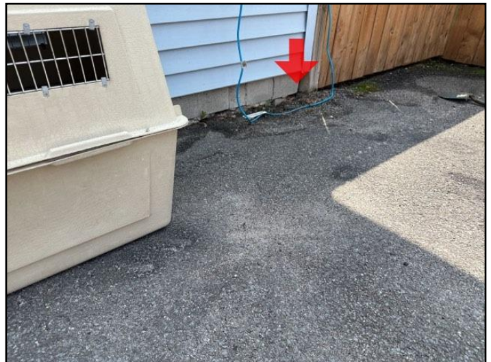
76. Improper slope or drainage
