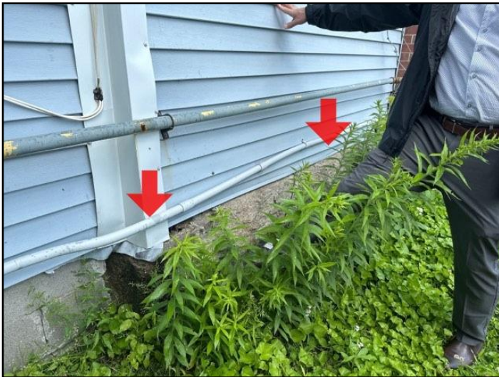
105. Spalling, crumbling or broken material
