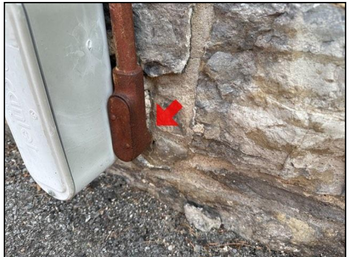
27. Caulking missing or ineffective
