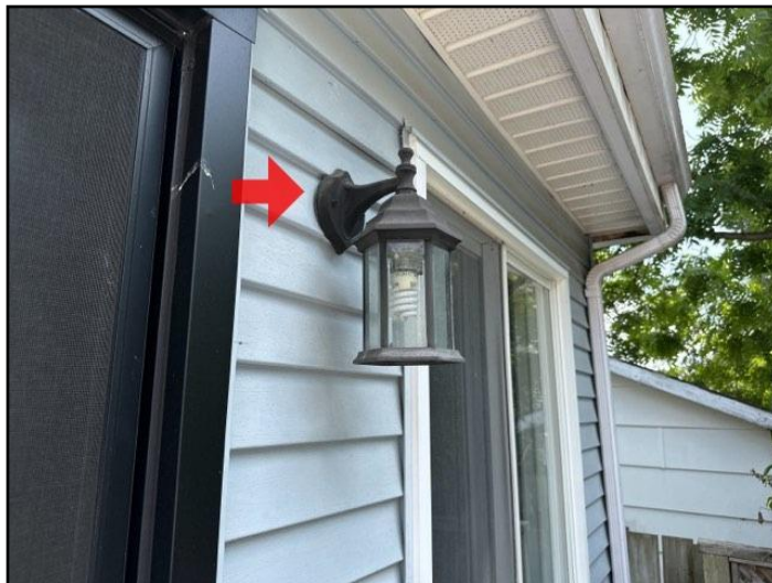
36. Caulking missing or ineffective
