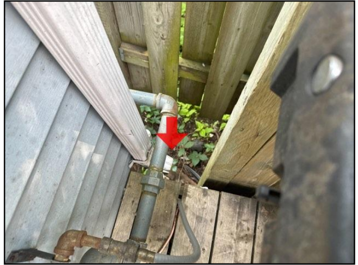
18. Should discharge 6 feet from building
