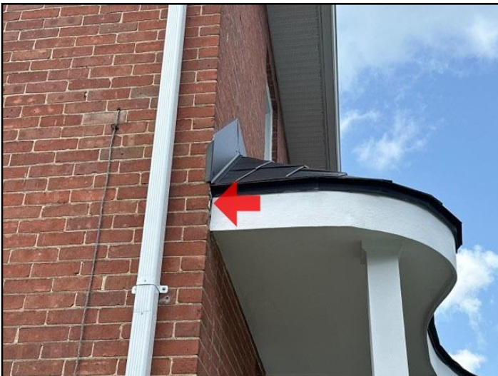
22. Caulking missing or ineffective
