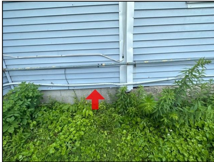
132. Not well secured
