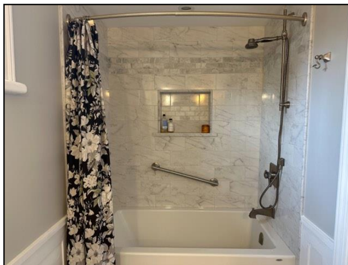
185. Caulking loose, missing or deteriorated
