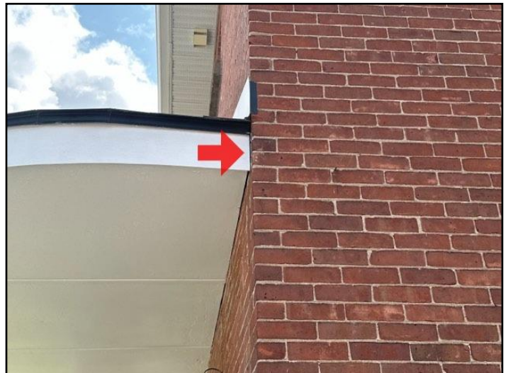
23. Caulking missing or ineffective
