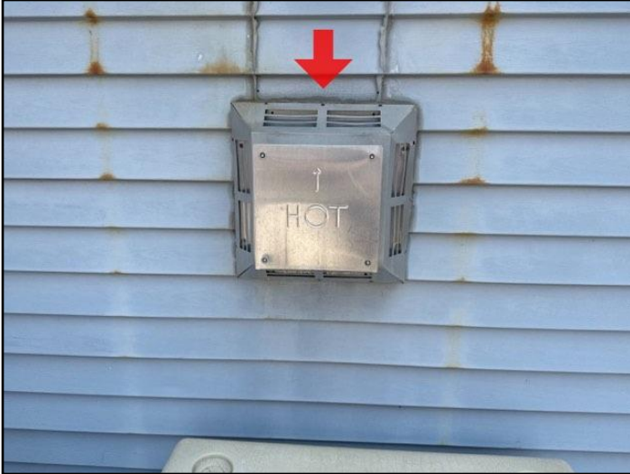
40. Loose or missing pieces
