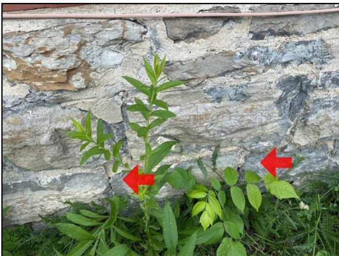
112. Mortar deteriorated or missing
