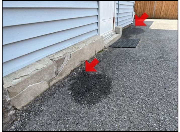
74. Improper slope or drainage
