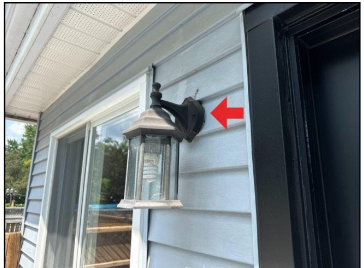
35. Caulking missing or ineffective
