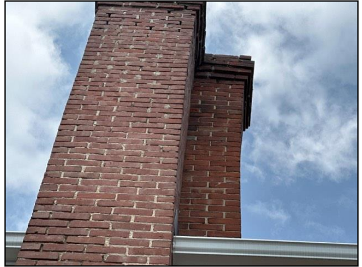
165. Loose, missing or deteriorated masonry
