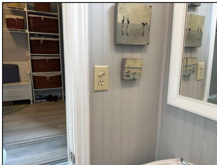
139. GFCI/GFI needed (Ground Fault Circuit...
