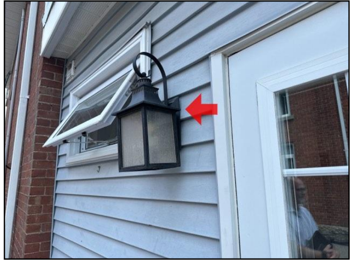
33. Caulking missing or ineffective
