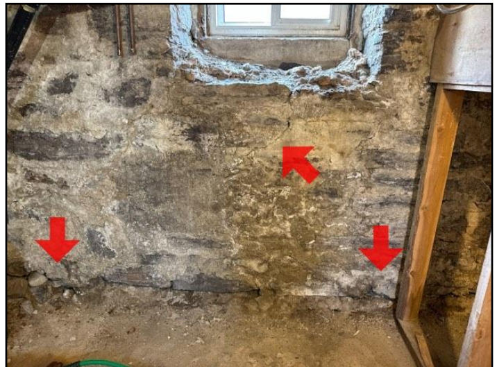
117. Mortar deteriorated or missing
