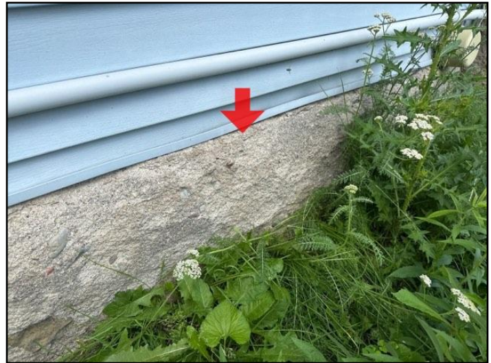
108. Spalling, crumbling or broken material
