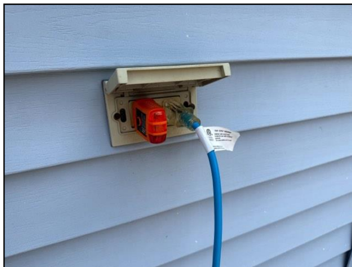
140. Test faulty on GFCI/GFI (Ground Fault...
