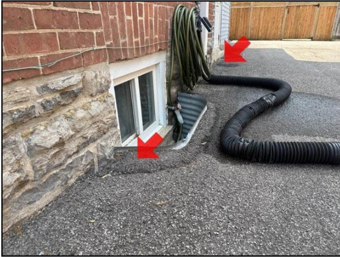
73. Improper slope or drainage
