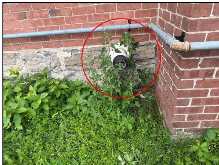
176. Rust, dirty, obstructed
