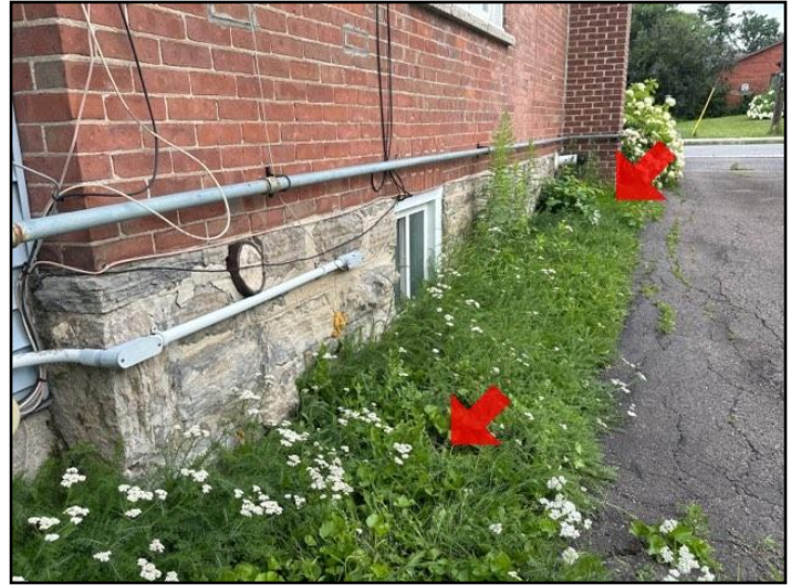
61. Improper slope or drainage
