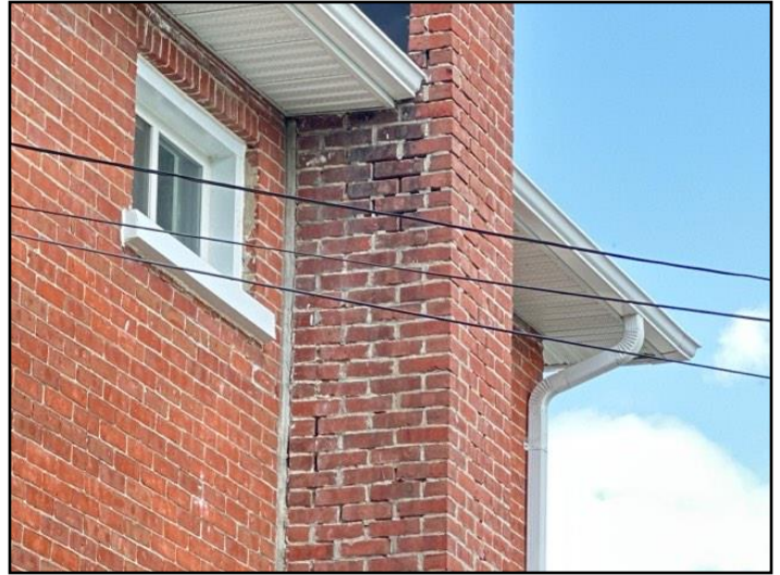
161. Loose, missing or deteriorated masonry
