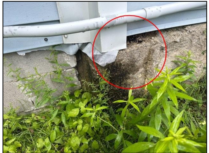
106. Spalling, crumbling or broken material
