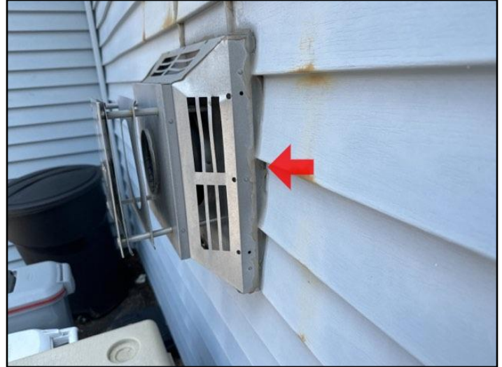
41. Loose or missing pieces
