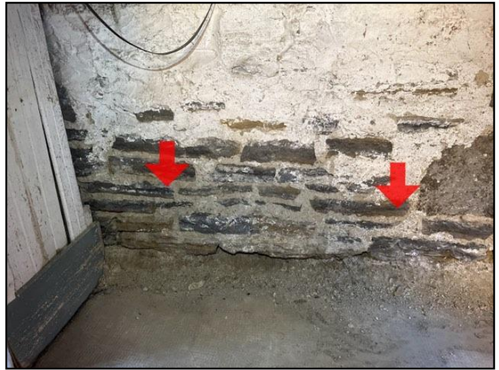
115. Mortar deteriorated or missing
