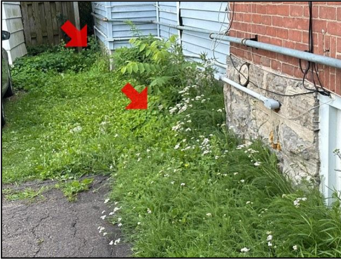
60. Improper slope or drainage
