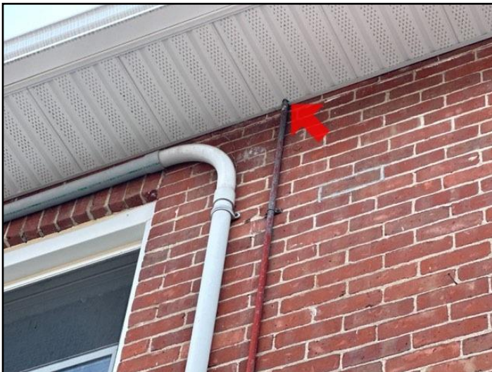
30. Caulking missing or ineffective
