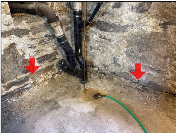
116. Mortar deteriorated or missing
