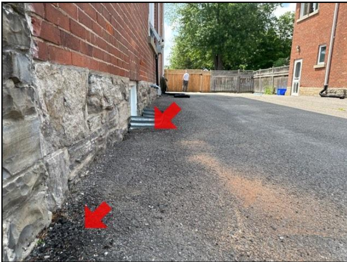
71. Improper slope or drainage
