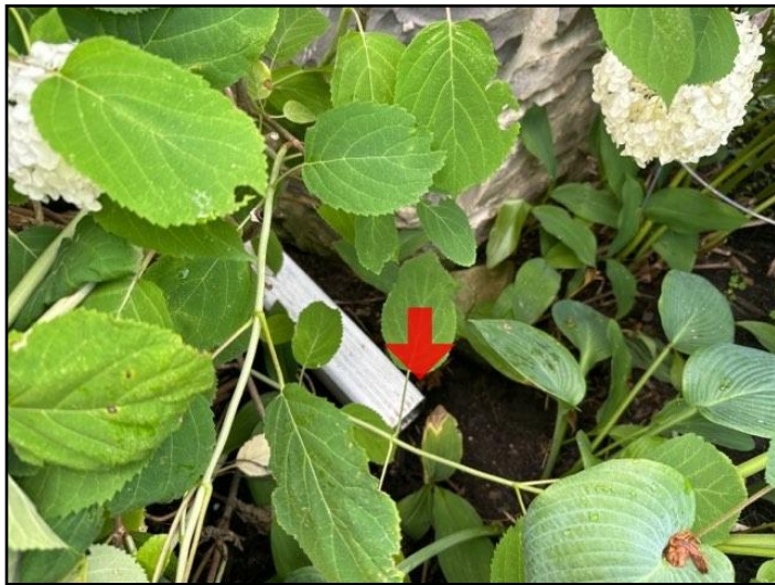
16. Should discharge 6 feet from building
