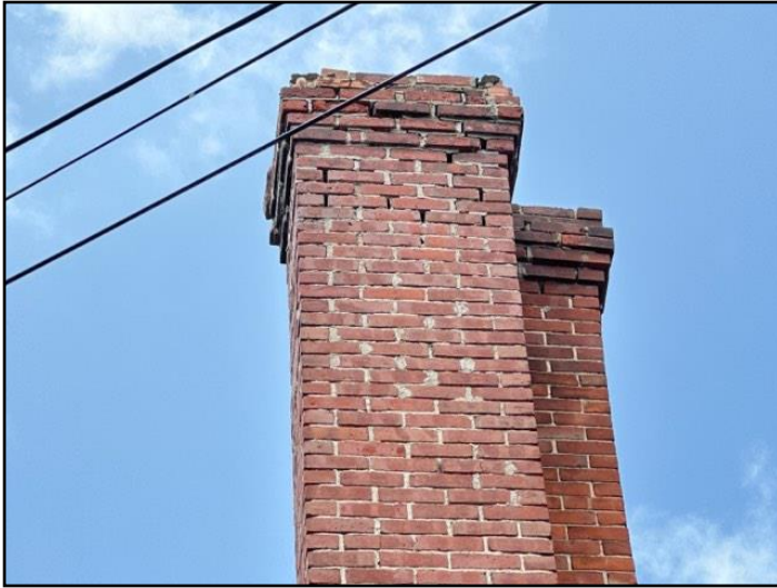
164. Loose, missing or deteriorated masonry
