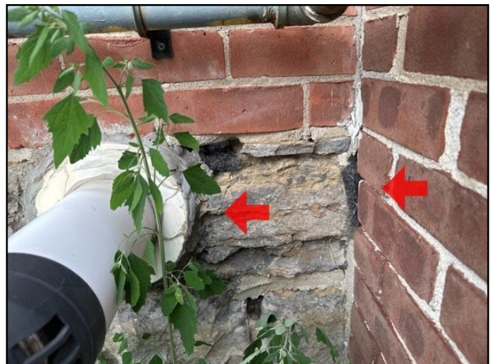
113. Mortar deteriorated or missing
