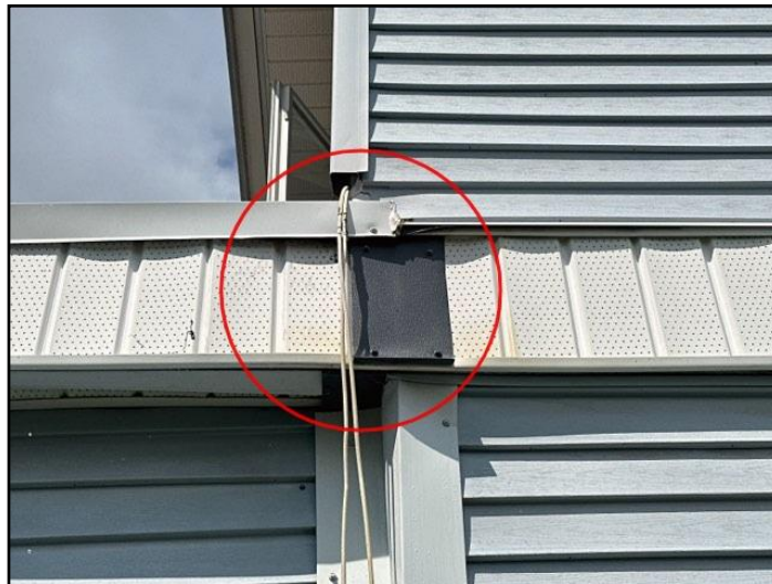
19. Loose or missing pieces
