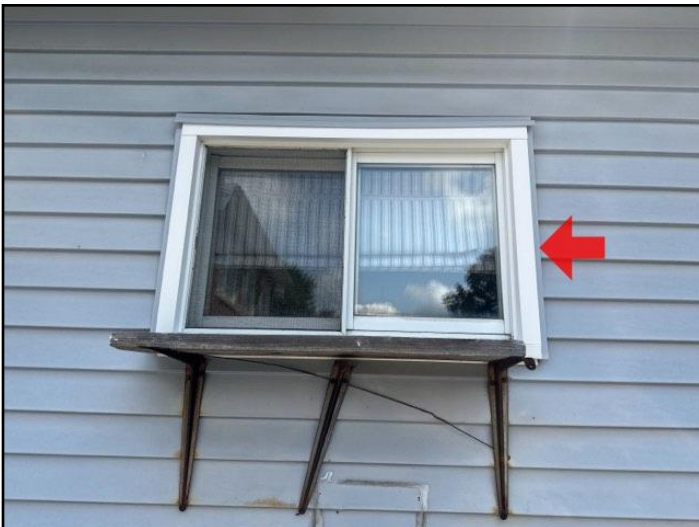
34. Caulking missing or ineffective
