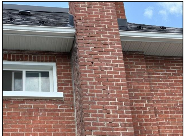
163. Loose, missing or deteriorated masonry
