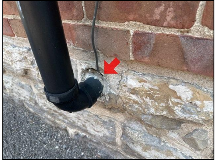
25. Caulking missing or ineffective
