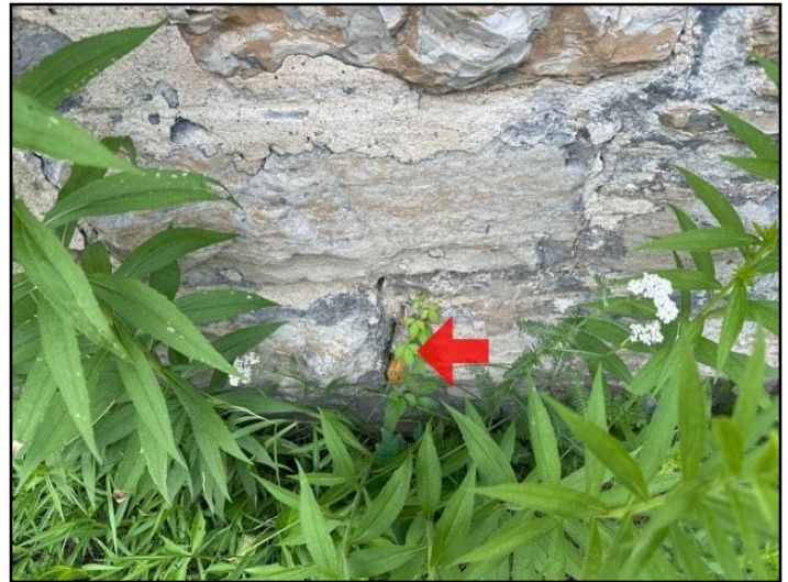
111. Mortar deteriorated or missing
