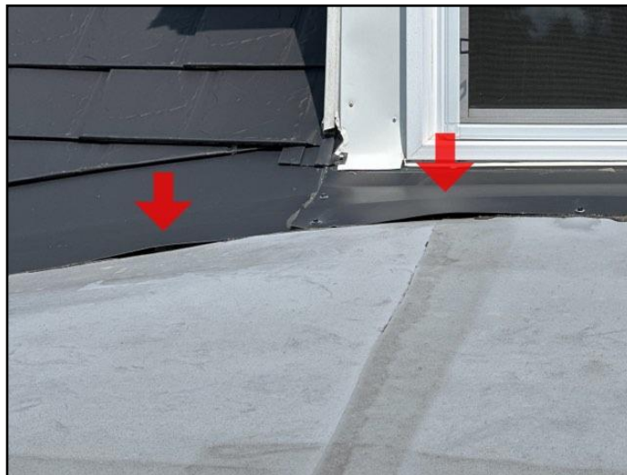
1. Valley flashing lifting
