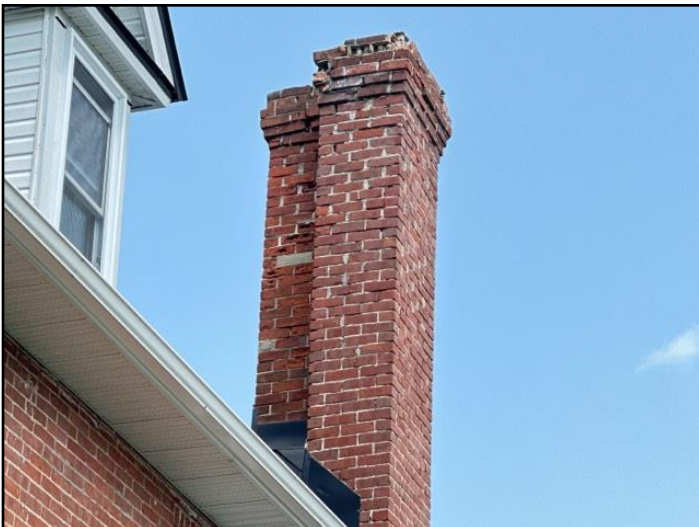
162. Loose, missing or deteriorated masonry
