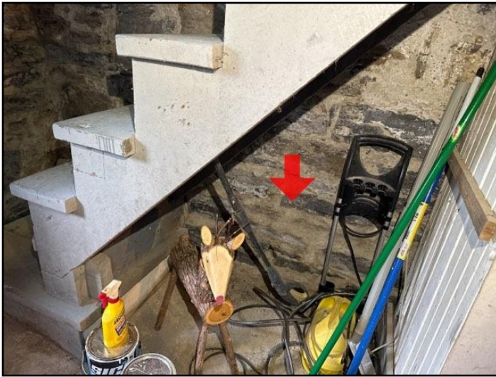
114. Mortar deteriorated or missing
