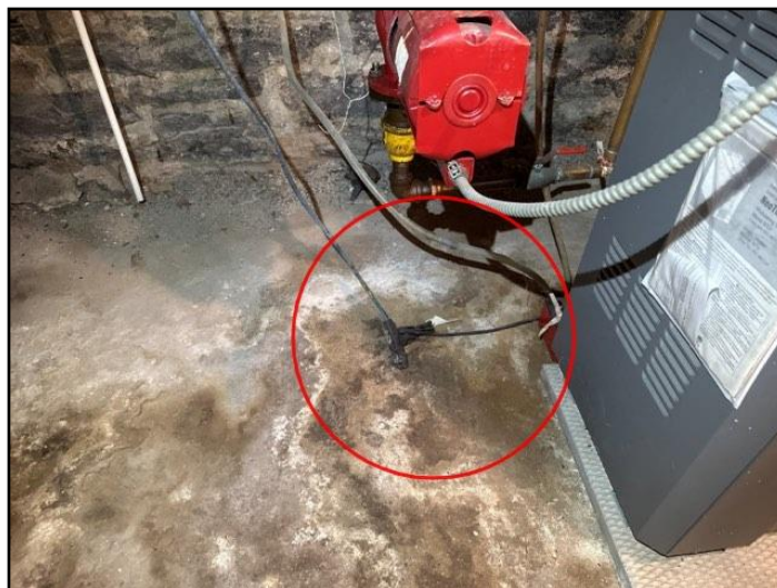
133. Extension cord used as permanent wiring
