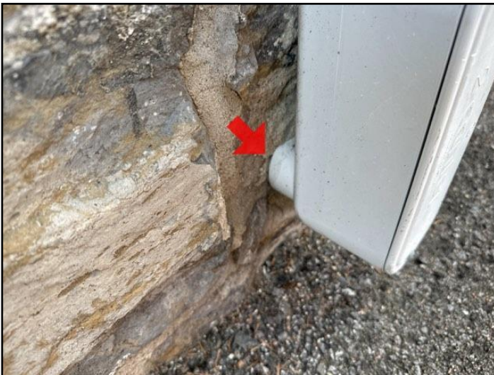
26. Caulking missing or ineffective
