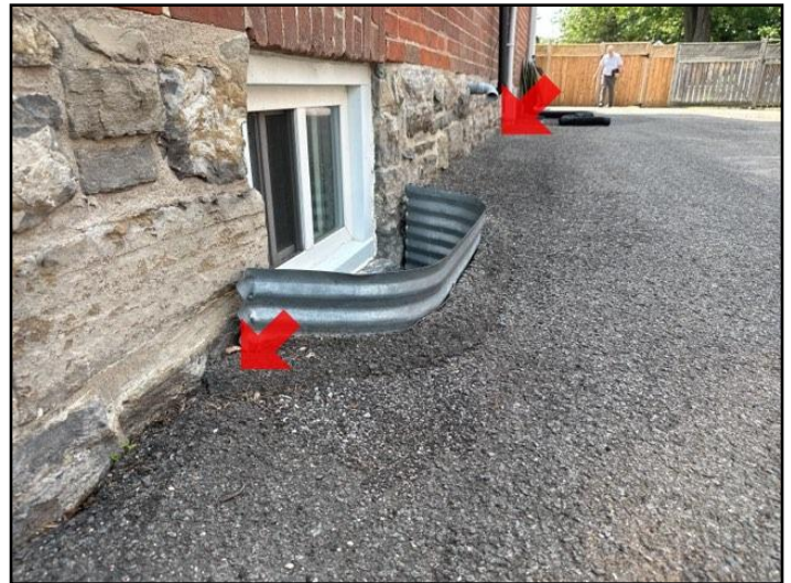
72. Improper slope or drainage
