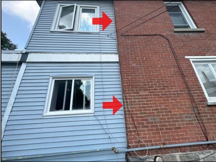
20. Caulking missing or ineffective
