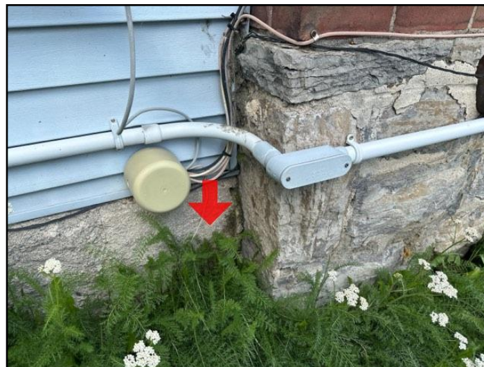
109. Spalling, crumbling or broken material
