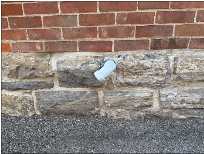
152. Rust, dirty, obstructed
