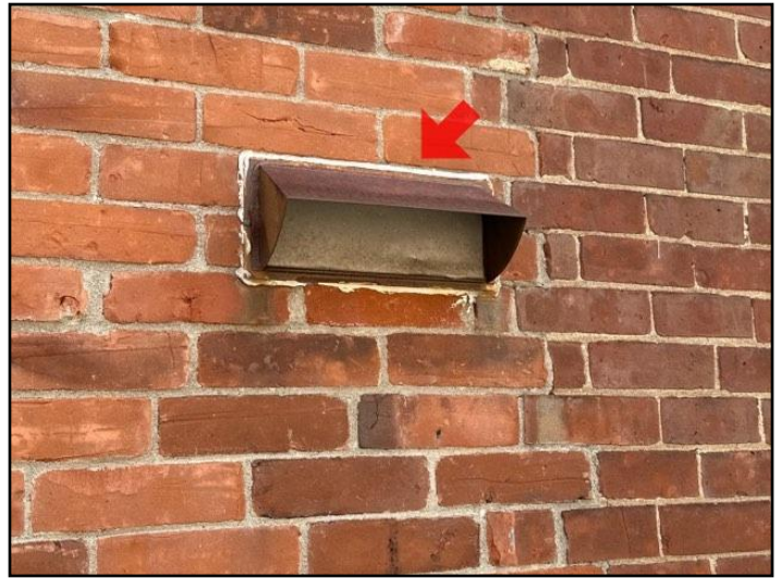
29. Caulking missing or ineffective
