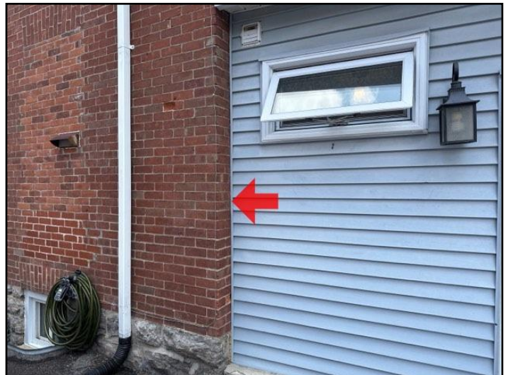
31. Caulking missing or ineffective
