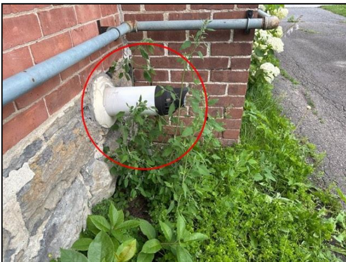
175. Rust, dirty, obstructed
