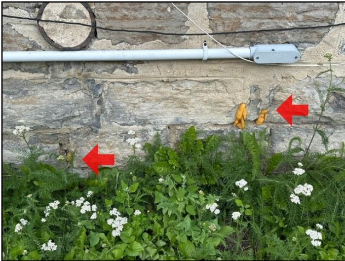
110. Mortar deteriorated or missing
