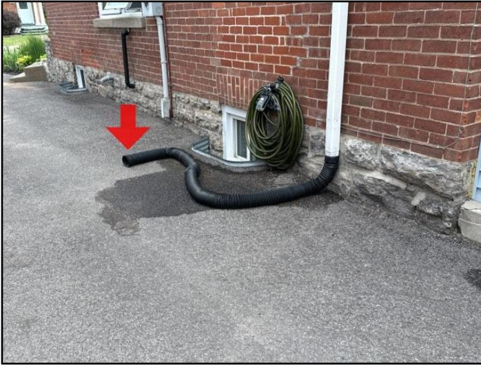
17. Should discharge 6 feet from building
