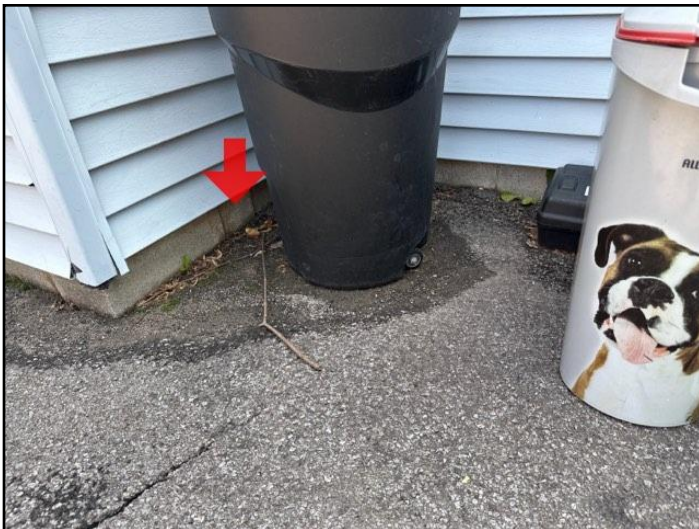
75. Improper slope or drainage
