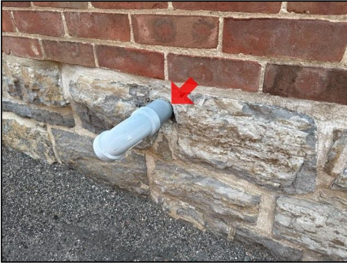
24. Caulking missing or ineffective
