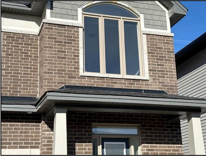
61. Debris on brick
