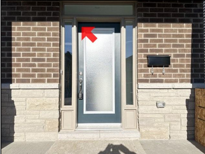
186. Weatherstripping missing or ineffective
