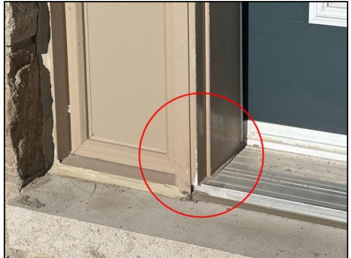
91. Damaged, cracked or loose
