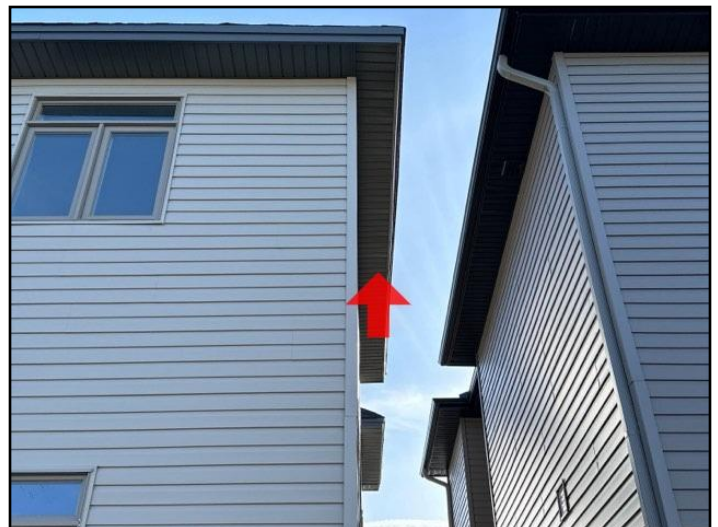
189. Does not discharge to exterior
