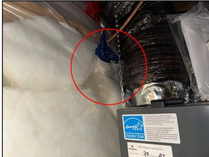
152. Loose, sagging or voids
