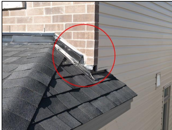
12. Damage, loose, open seams, patched
