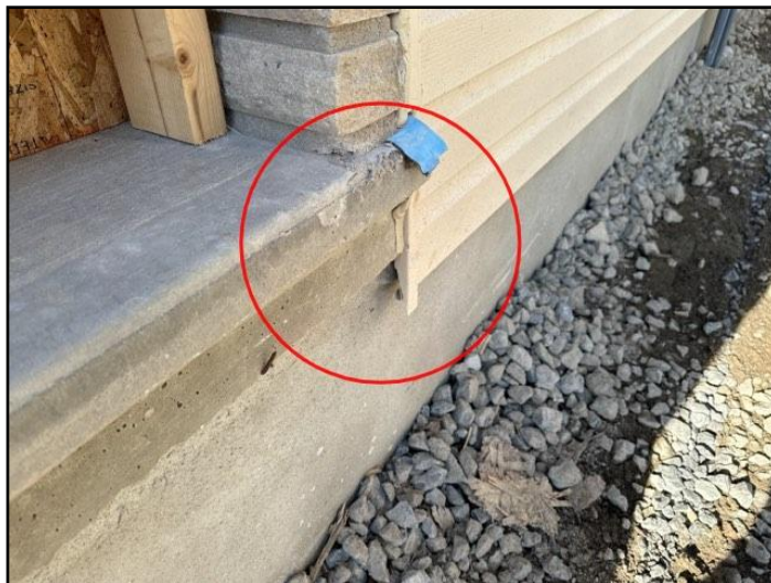
23. Caulking missing or ineffective
