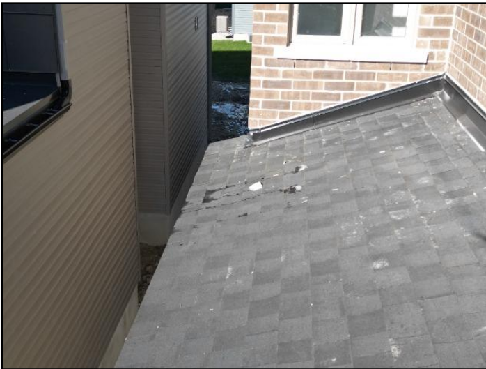
4. Remove all loose debris from roof coverings.
