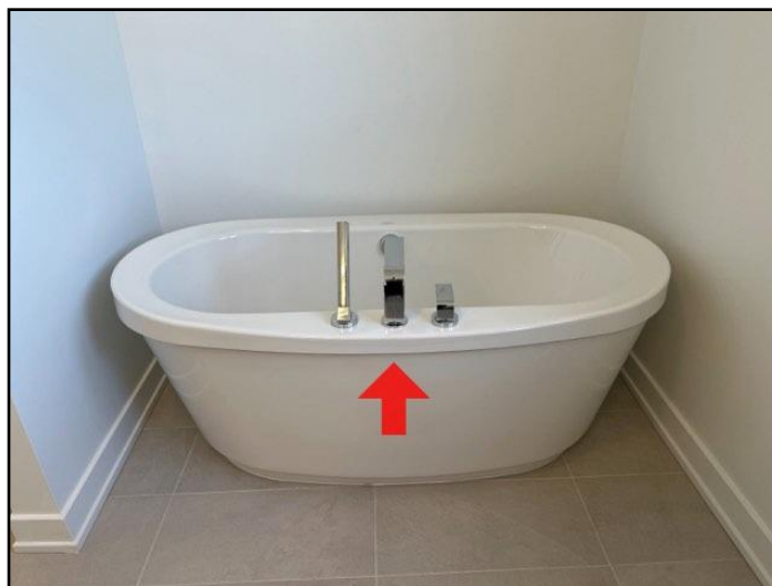
171. Loose or unstable
