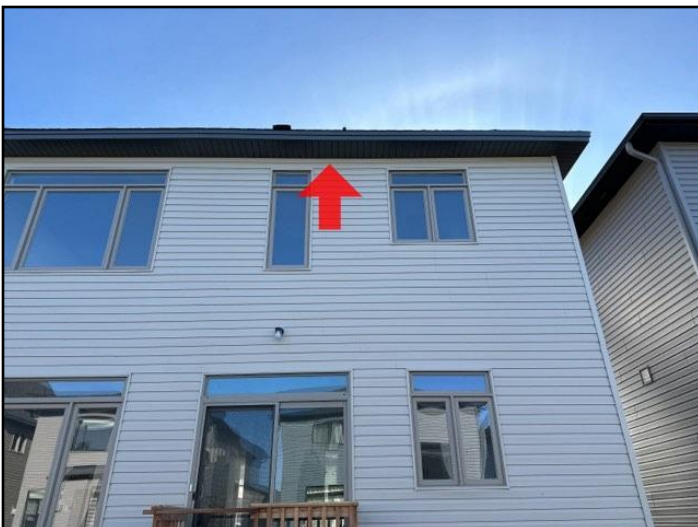
188. Does not discharge to exterior
