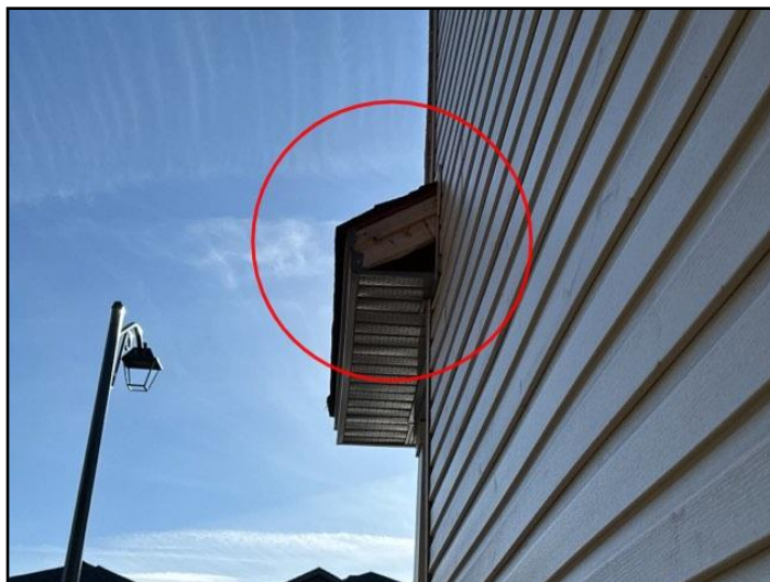
17. Loose or missing pieces
