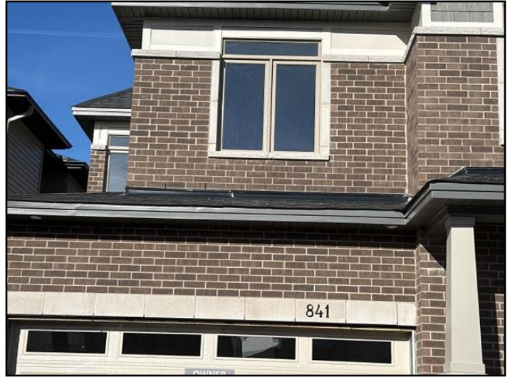
62. Debris on brick
