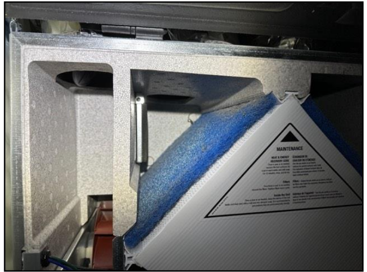
147. Dirt in cabinet
