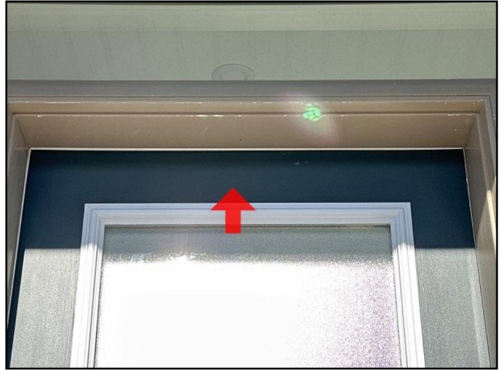
93. Damaged, cracked or loose
