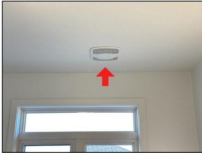
190. Does not discharge to exterior
