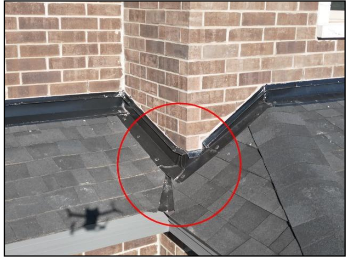
11. Damage, loose, open seams, patched
