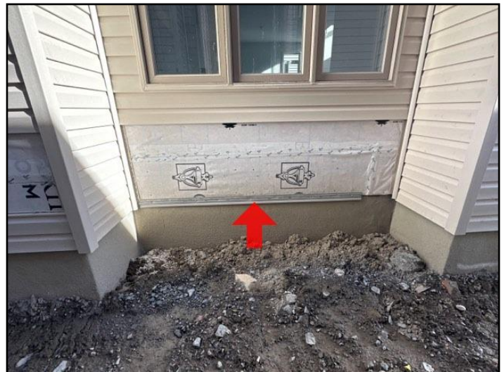
27. Loose or missing pieces
