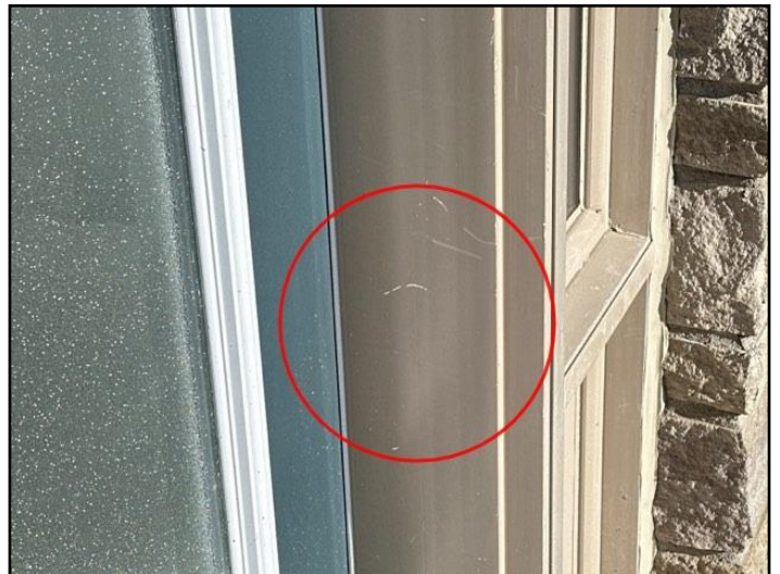
95. Damaged, cracked or loose
