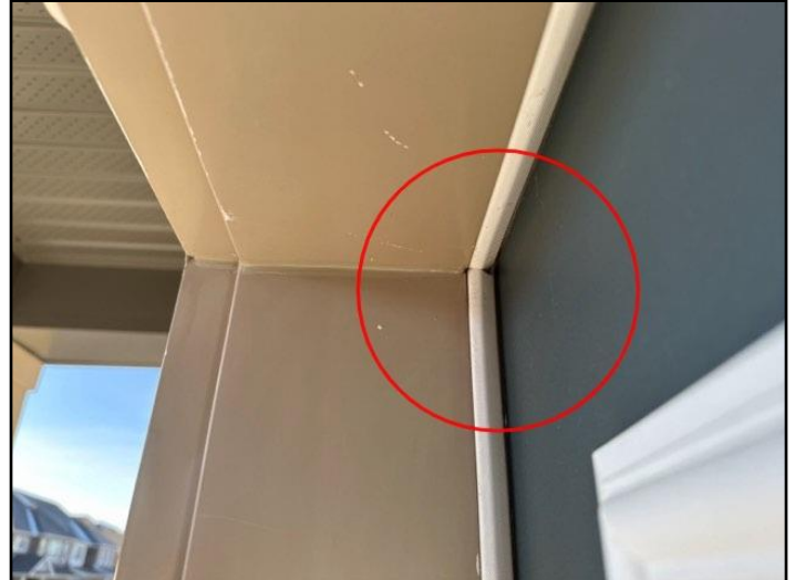
187. Weatherstripping missing or ineffective
