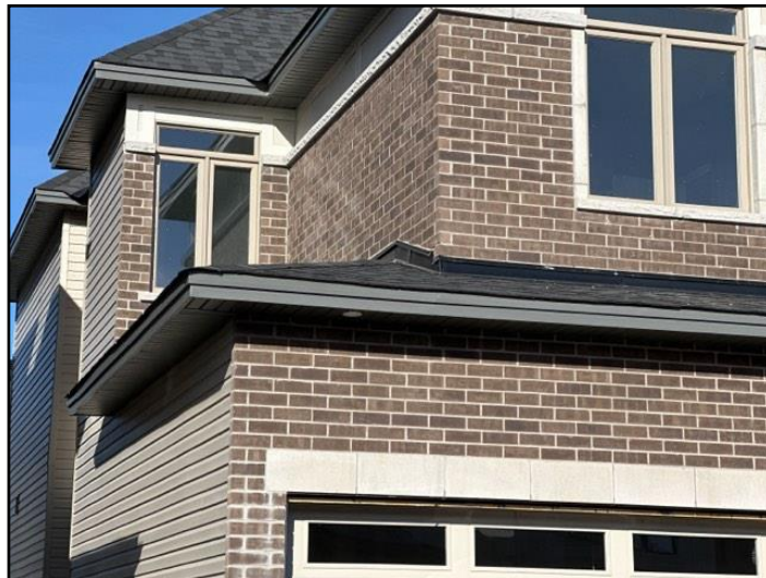
63. Debris on brick
