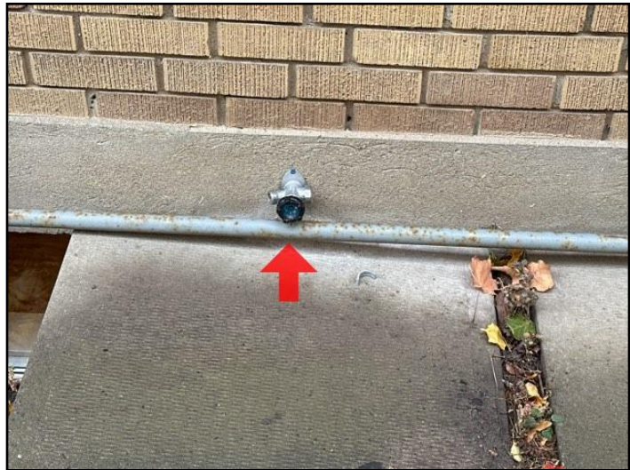
93. Poor slope on frost-free bib/bibb (outdoor...)
