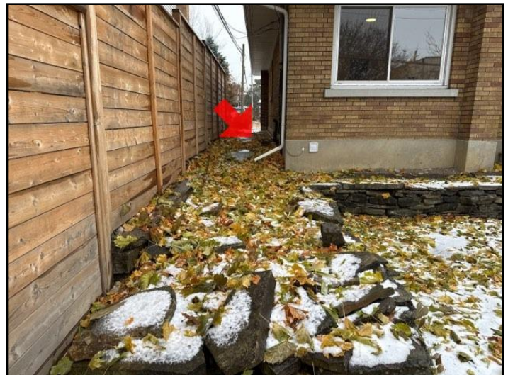
24. Improper slope or drainage
