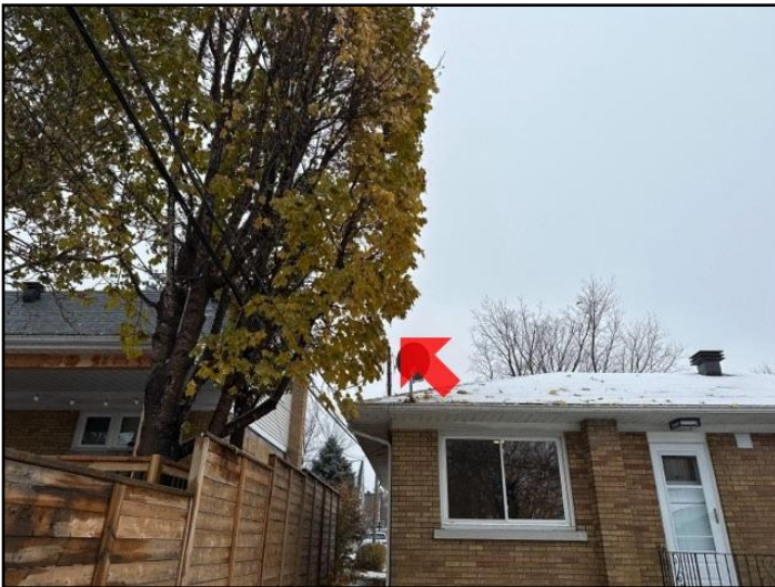
21. Trees or shrubs too close to building
