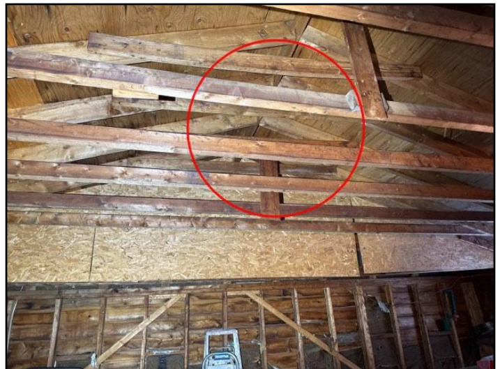
45. Too small or overspanned
