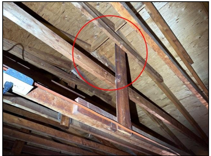
43. Too small or overspanned
