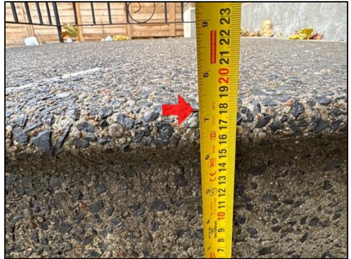
18. Stair rise too big or not uniform
