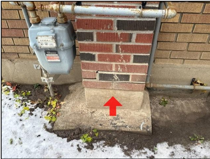
76. Settling or leaning
