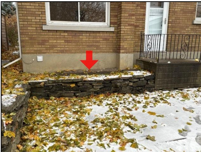
23. Improper slope or drainage
