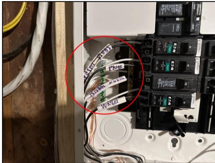
51. Sheathing not removed
