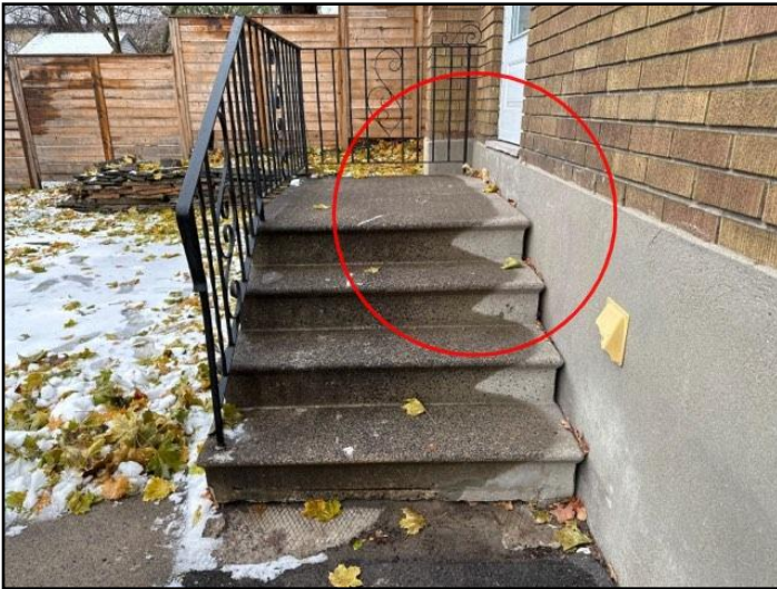
17. Stair rise too big or not uniform
