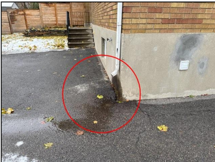
3. Should discharge 6 feet from building
