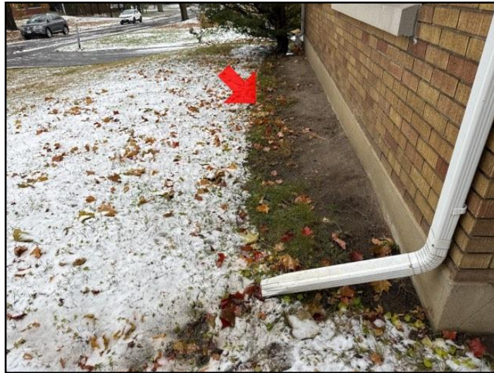
25. Improper slope or drainage
