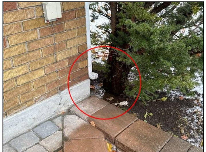
4. Should discharge 6 feet from building
