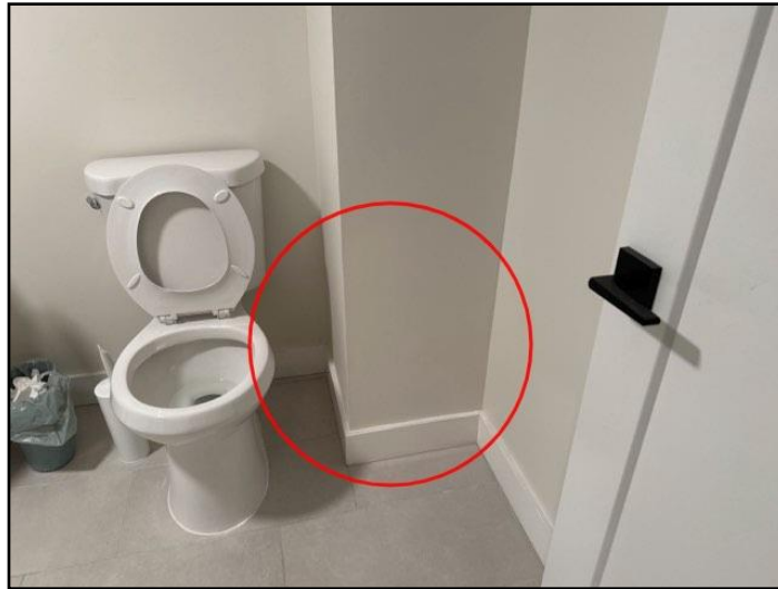
90. Clean-outs missing or inaccessible
