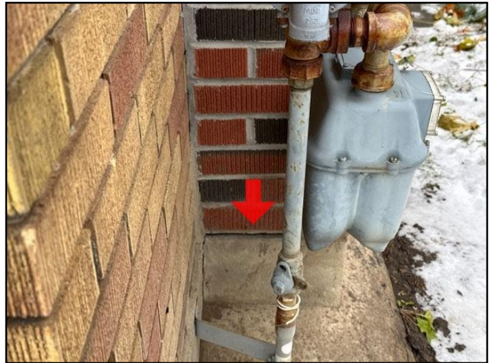
77. Settling or leaning
