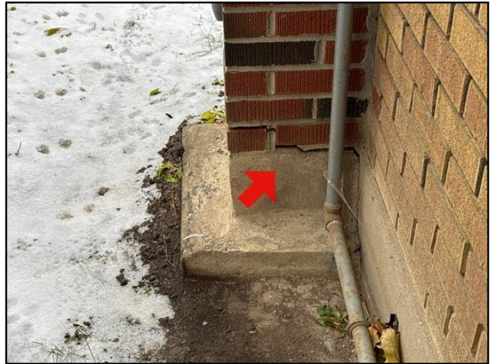
75. Settling or leaning
