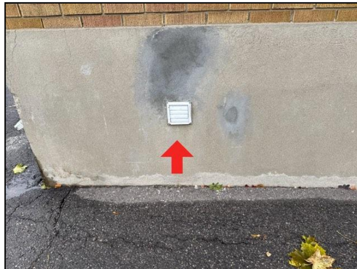
97. Clean dryer vent
