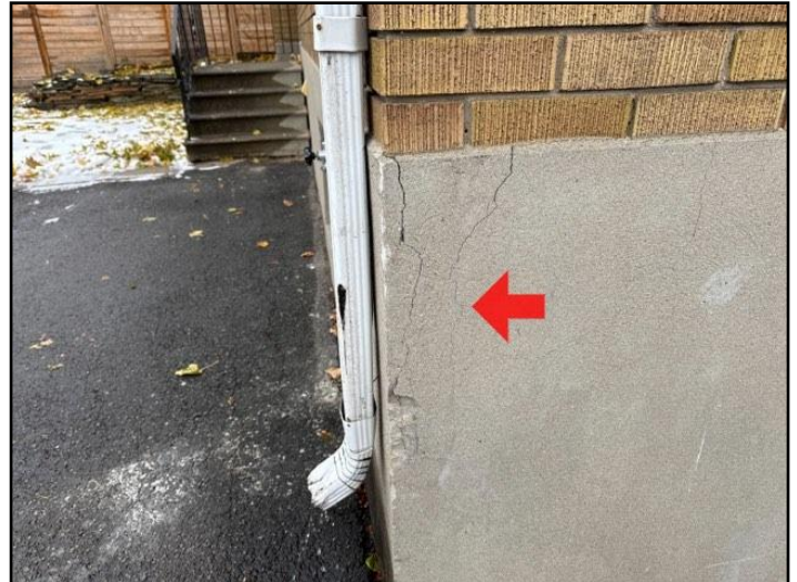
10. Parging damaged or missing
