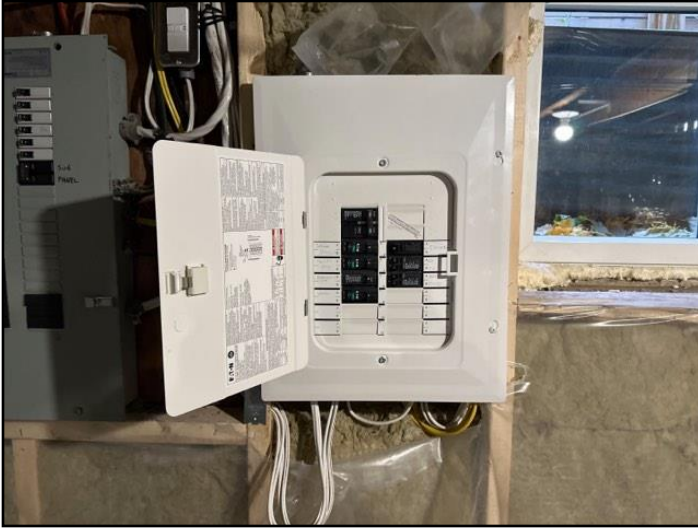
52. Modified or added wiring
