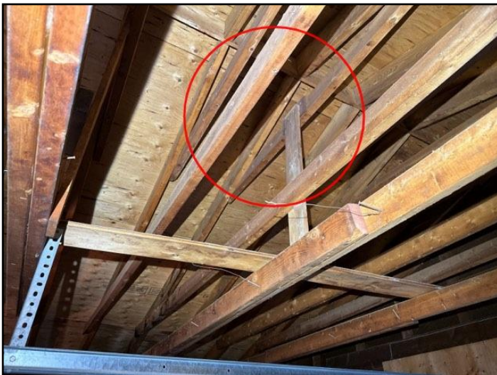
44. Too small or overspanned
