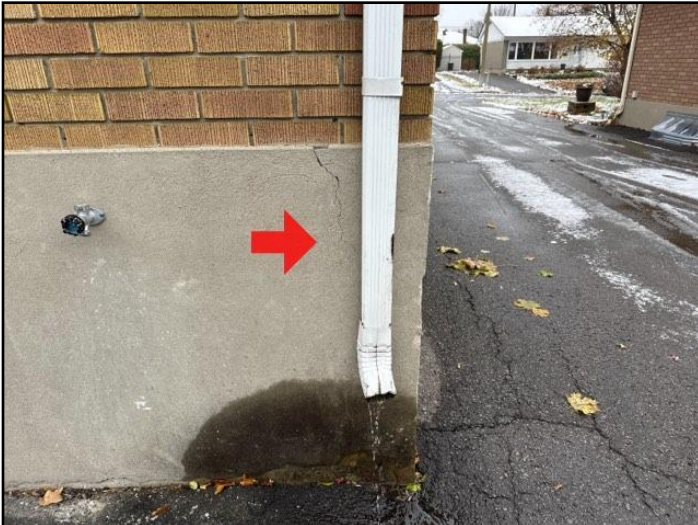
9. Parging damaged or missing
