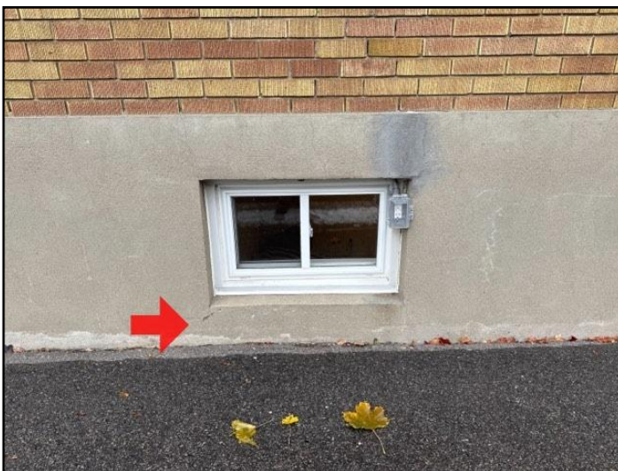
40. Typical minor cracks
