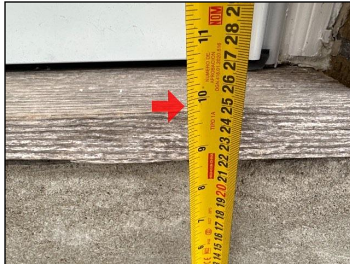
19. Stair rise too big or not uniform
