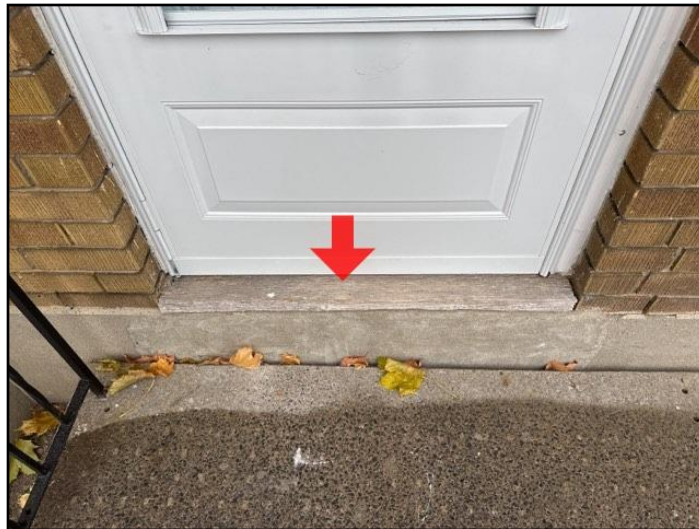
15. Paint or stain needed
