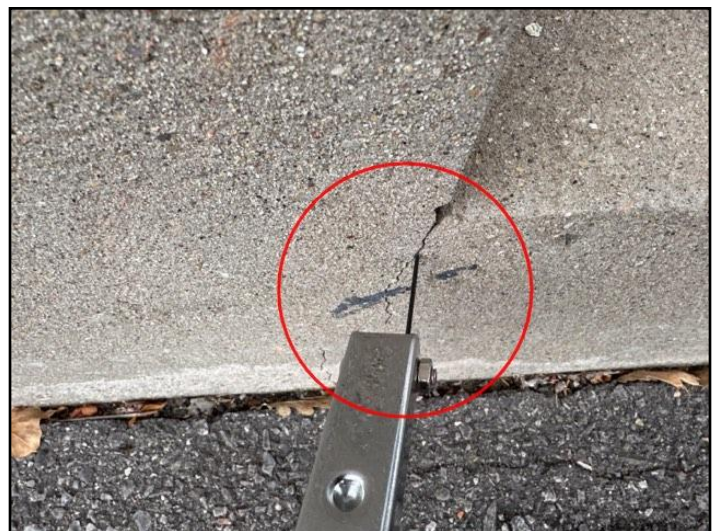
41. Typical minor cracks
