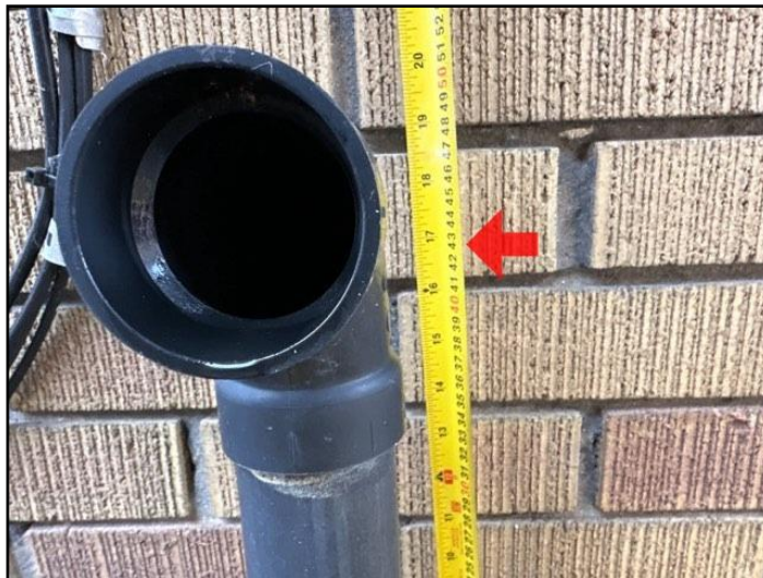
72. Exhaust vent missing insulation
