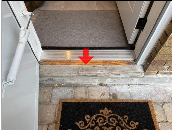
16. Paint or stain needed
