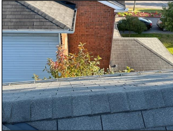
24. Trees or shrubs too close to building
