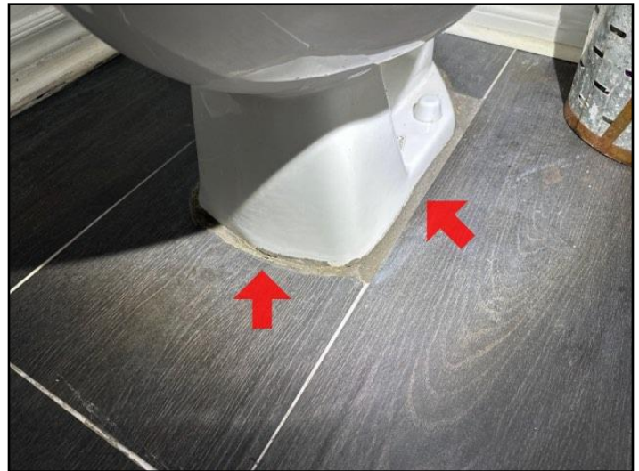
95. Floor damage suspected
