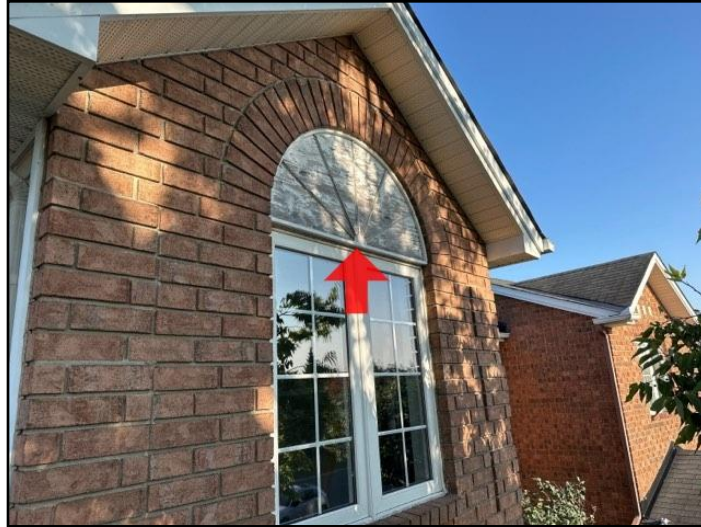
10. Paint or stain needed
