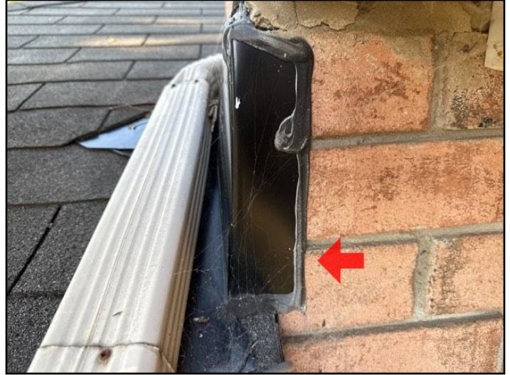
6. Damage, loose, open seams, patched
