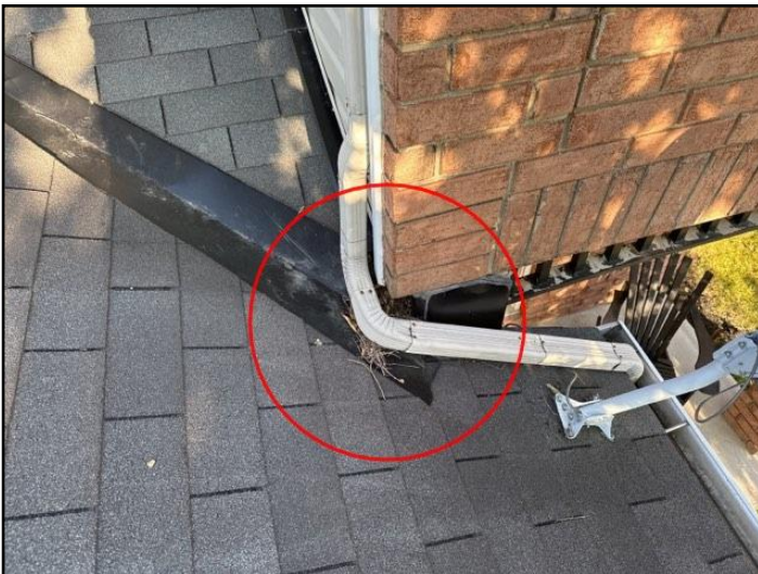
3. Wood joints break into valley
