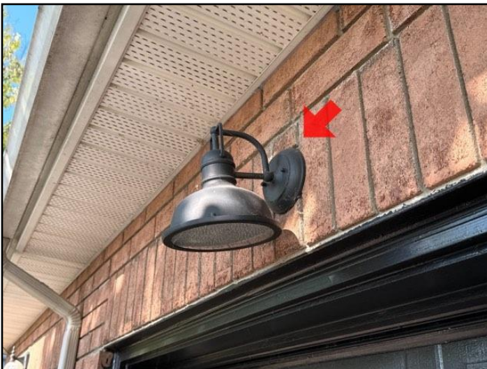
11. Caulking missing or ineffective
