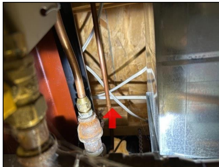
55. Modified or added wiring
