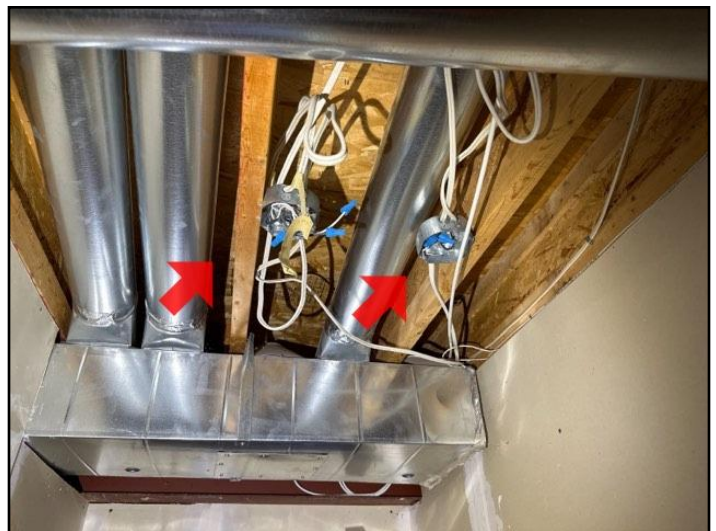
52. Modified or added wiring
