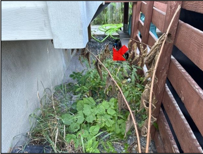
27. Improper slope or drainage
