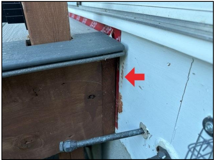
17. No step up into building
