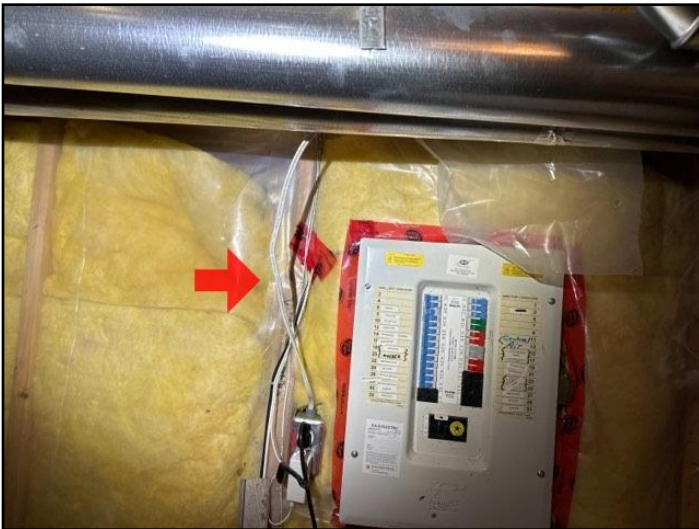
47. Modified or added wiring
