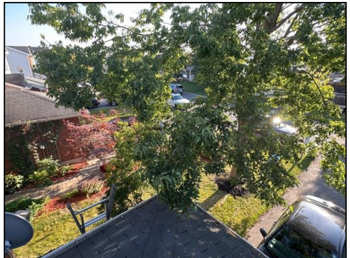
23. Trees or shrubs too close to building
