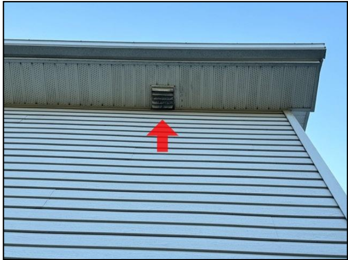
9. Vents - ineffective / missing
