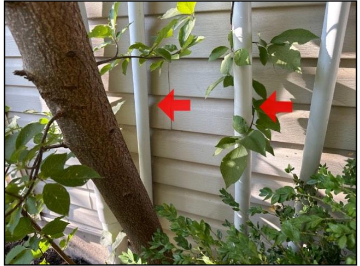
44. Conduit or cable damaged
