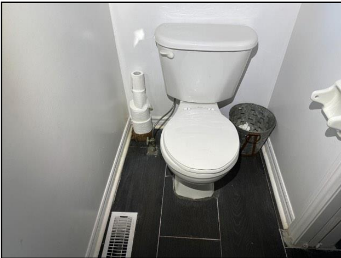
94. Floor damage suspected
