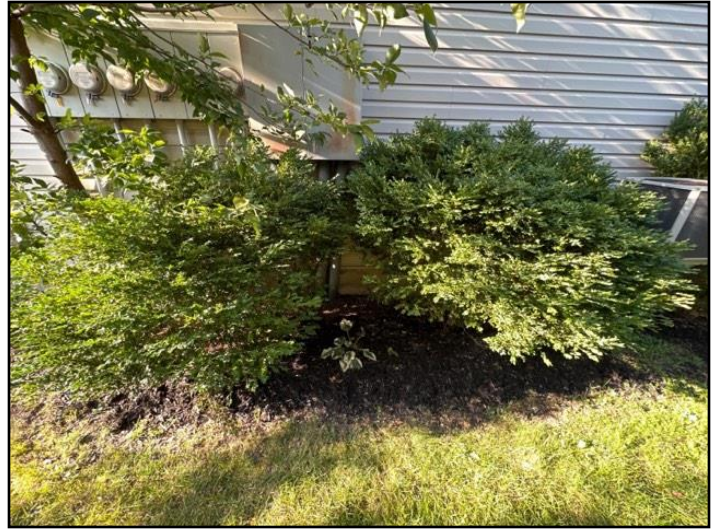
21. Trees or shrubs too close to building
