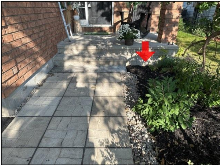
25. Improper slope or drainage
