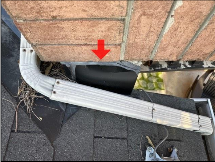
5. Damage, loose, open seams, patched
