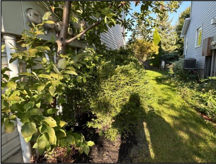
20. Trees or shrubs too close to building
