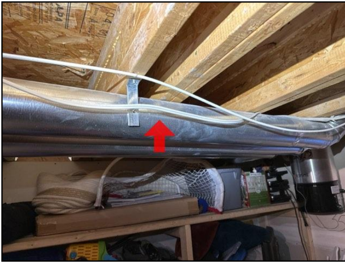
49. Modified or added wiring
