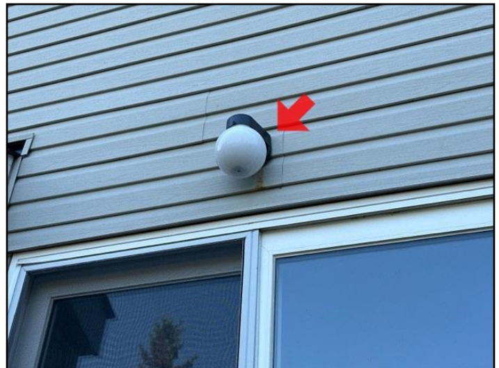
12. Caulking missing or ineffective
