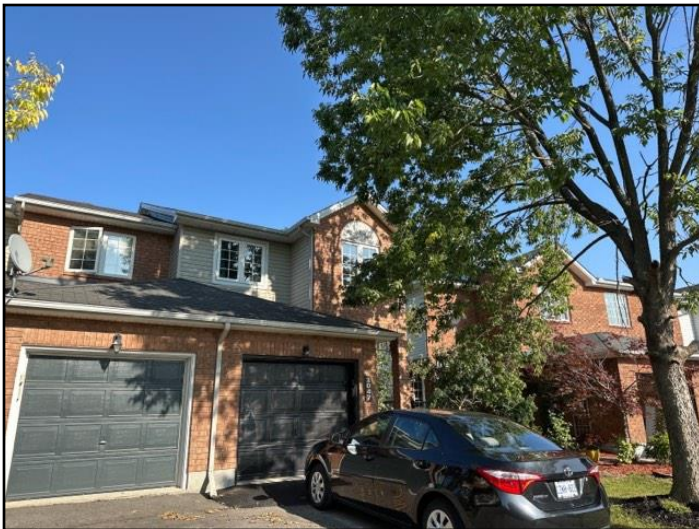
18. Trees or shrubs too close to building
