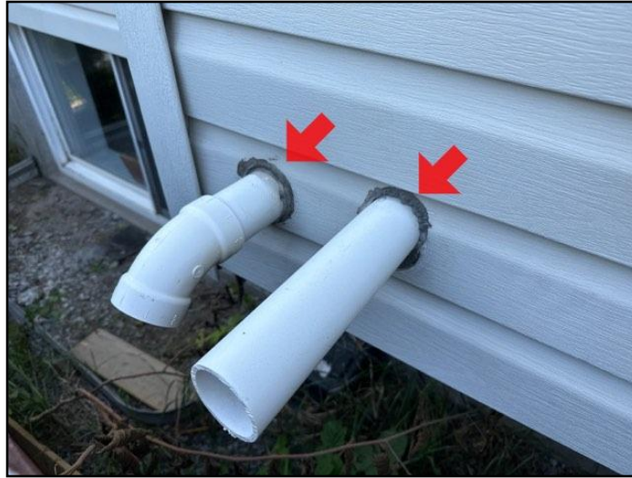
13. Caulking missing or ineffective
