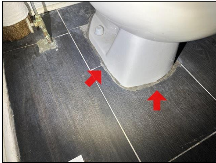
96. Floor damage suspected
