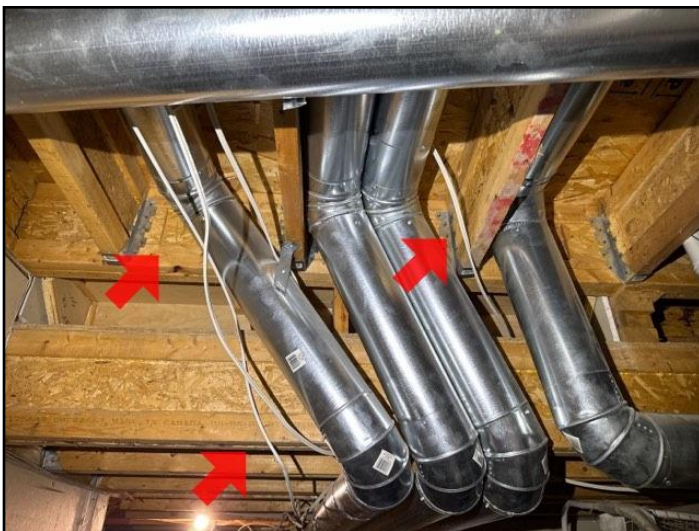
51. Modified or added wiring
