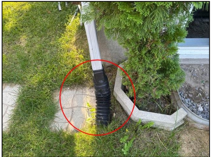
8. Should discharge 6 feet from building
