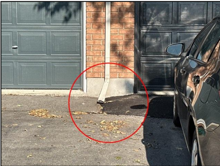
7. Should discharge 6 feet from building
