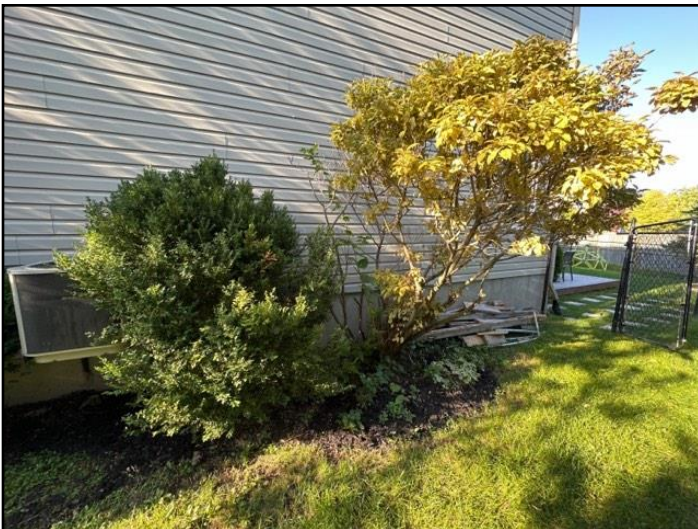
22. Trees or shrubs too close to building
