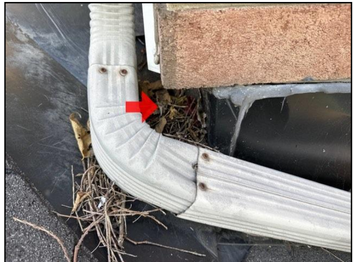
4. Wood joints break into valley
