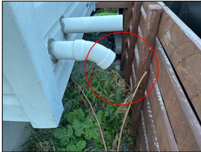
84. Rust, dirty, obstructed
