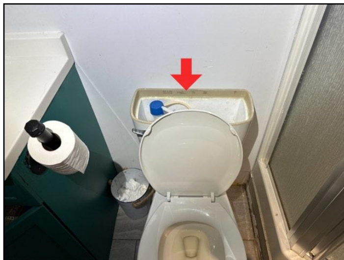
97. Broken or cracked tank lids, bowls or seats
