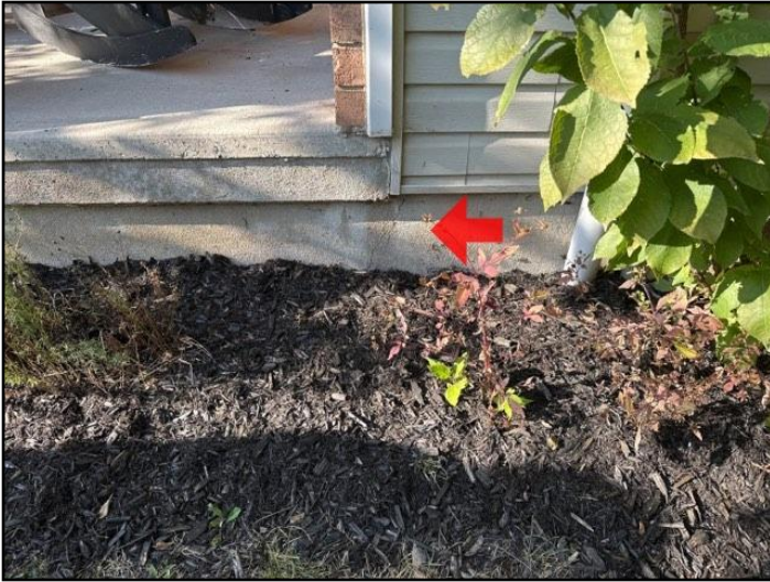
41. Typical minor cracks
