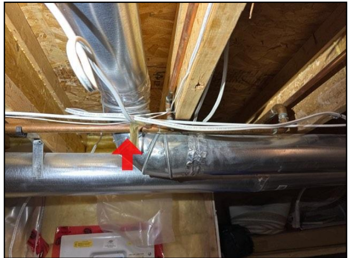
48. Modified or added wiring
