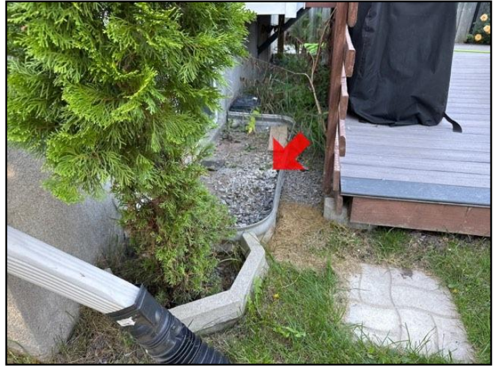
28. Improper slope or drainage
