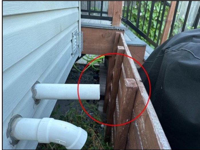
72. Rust, dirty, obstructed
