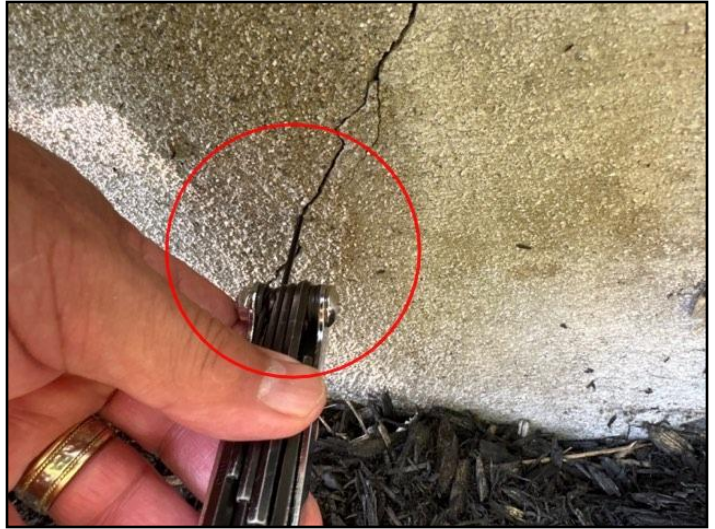
42. Typical minor cracks
