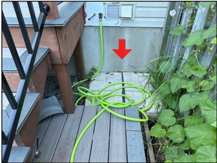
26. Improper slope or drainage
