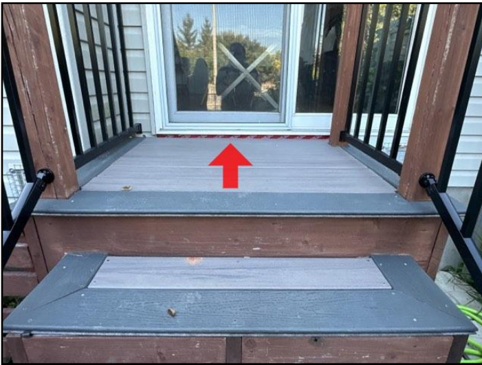
16. No step up into building
