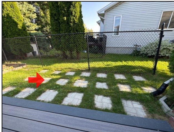
29. Improper slope or drainage
